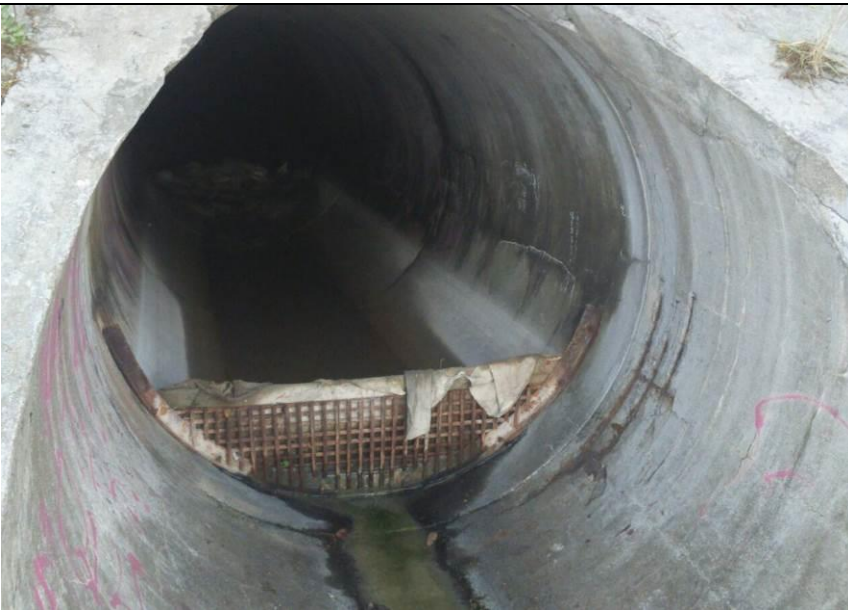
Outfall 1: Clean water is discharging.
