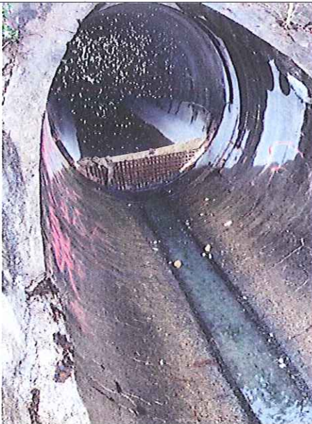
Outfall 1: Clean water is discharging.
