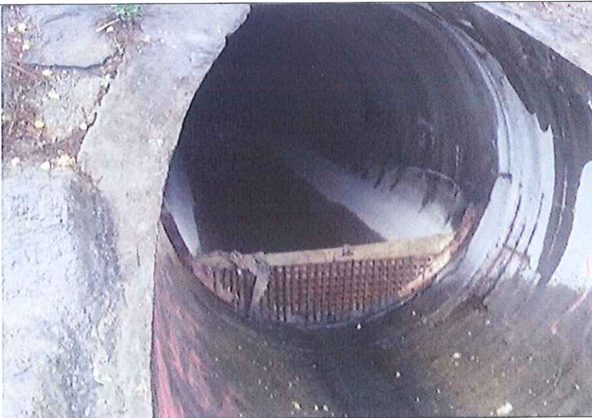
Outfall 1: Clean water is discharging.
