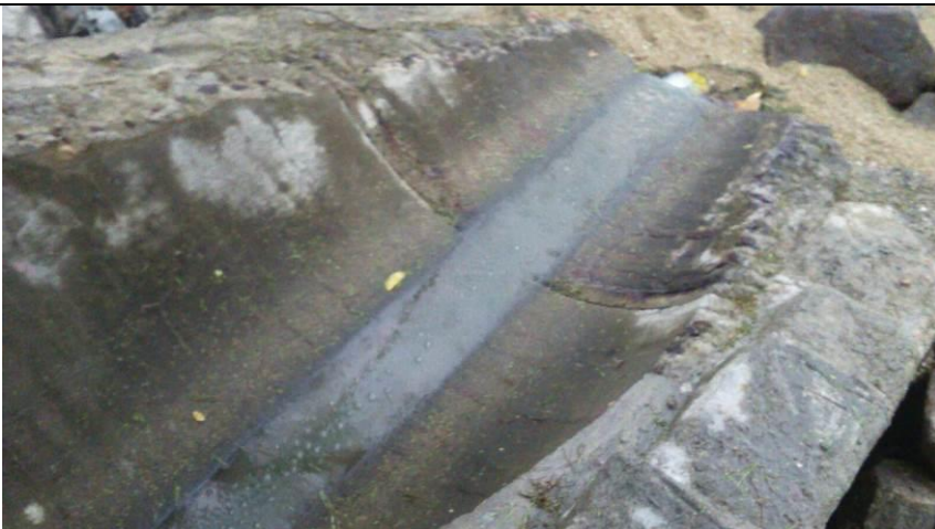
Outfall 1: Clean water is discharging.
