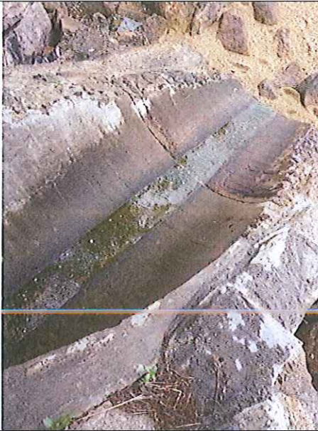
Outfall 1: Clean water is discharging.
