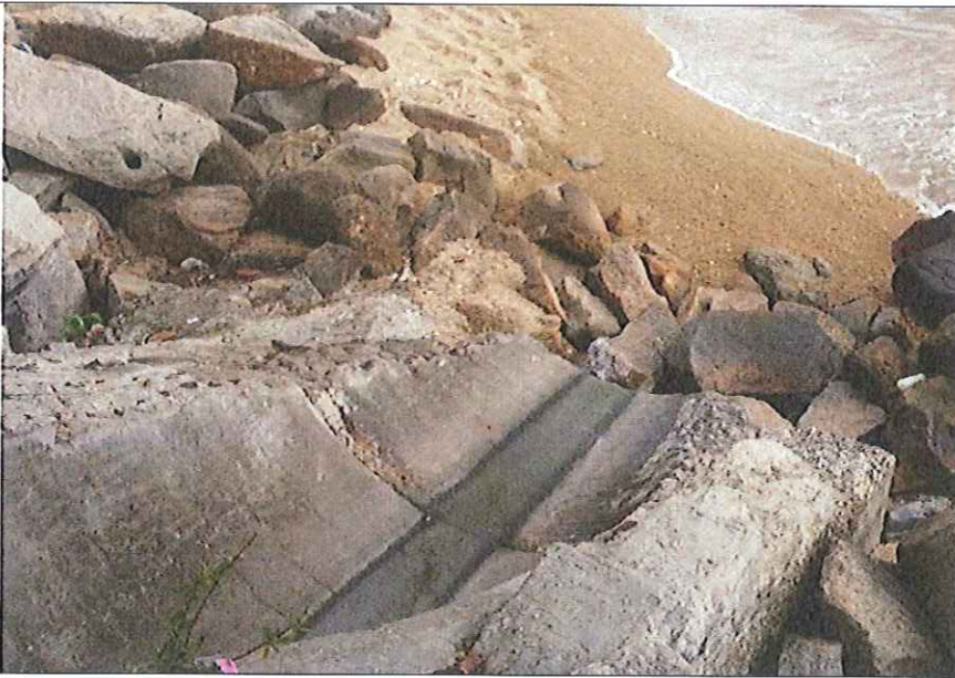
Outfall 1: Clean water is discharging.
