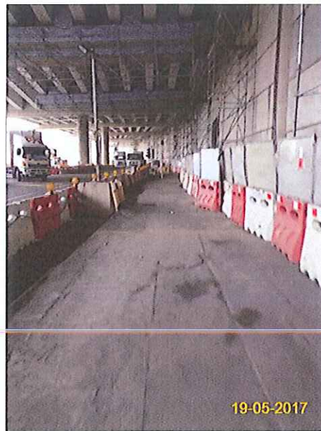
Item 5. Hoarding with panel around works area & Item 6. Temporary traffic management lighting.
