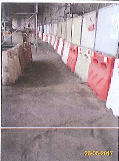
Item 5. Hoarding with panel around works area & Item 6. Temporary traffic management lighting.
