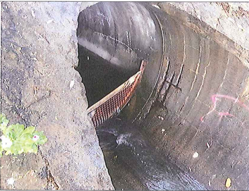
Outfall 1: Clean water is discharging.
