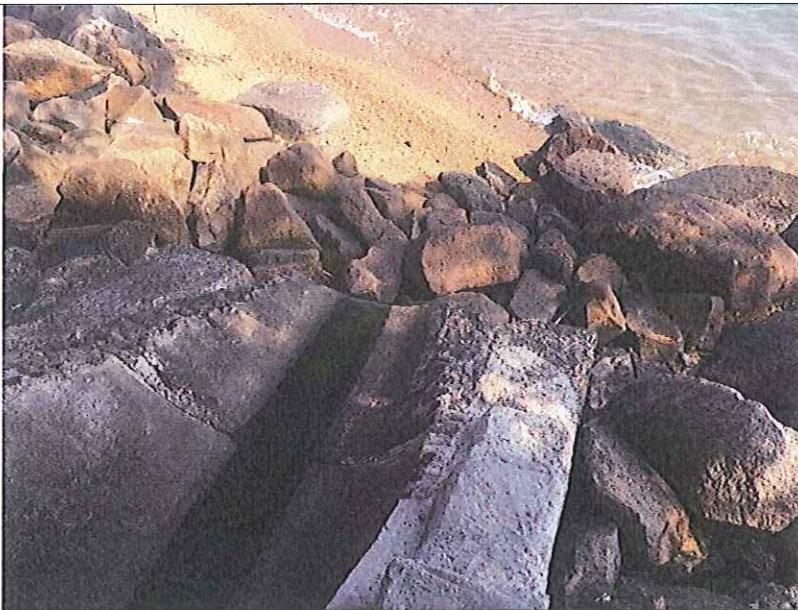
Outfall 1: Clean water is discharging.
