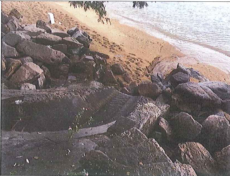
Outfall 1: Clean water is discharging.
