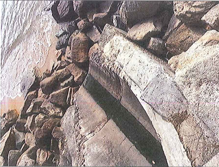
Outfall 1: Clean water is discharging.
