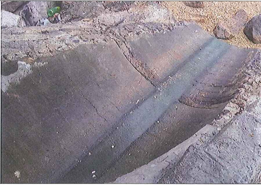
Outfall 1: Clean water is discharging.
