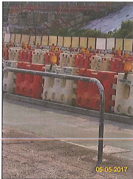
Item 5. Hoarding with panel around works area & Item 6. Temporary traffic management lighting.
