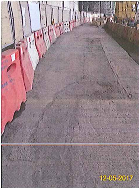
Item 5. Hoarding with panel around works area & Item 6. Temporary traffic management lighting.
