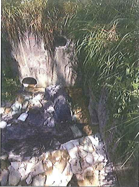
Stream B Outfall: No water is discharging.
