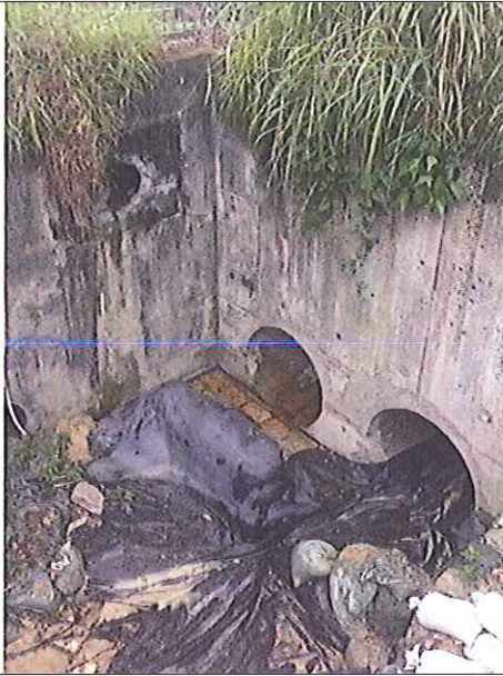
Stream B Outfall: No water is discharging.
