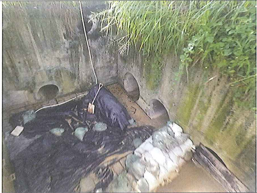
Stream B Outfall: No water is discharging.
