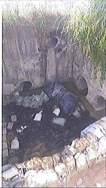
Stream B Outfall: No water is discharging.
