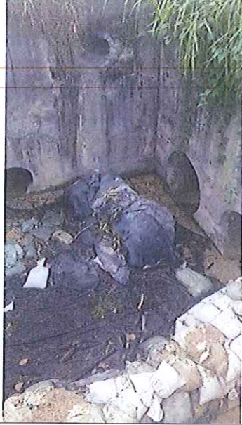
Stream B Outfall: No water is discharging.
