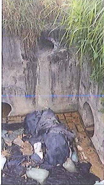
Stream B Outfall: No water is discharging.
