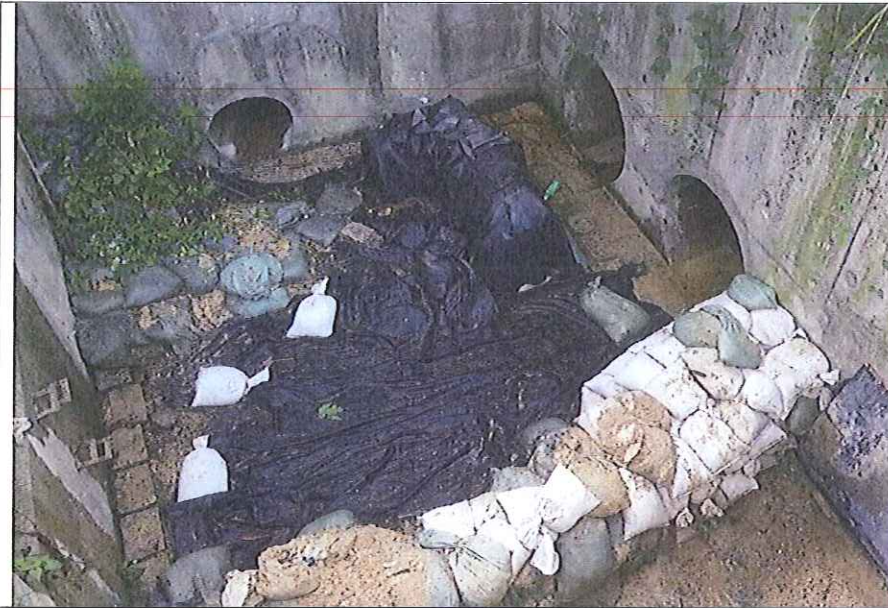
Stream B Outfall: No water is discharging.
