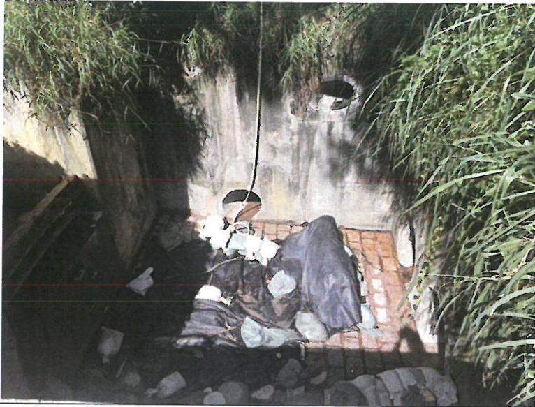
Stream B Outfall: No water is discharging.
