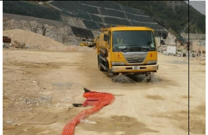
Photo 2 Watering of haul road by water truck to keep road surface wet
