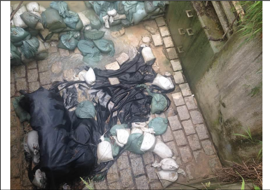
Stream B Outfall: Clean water is discharging.
