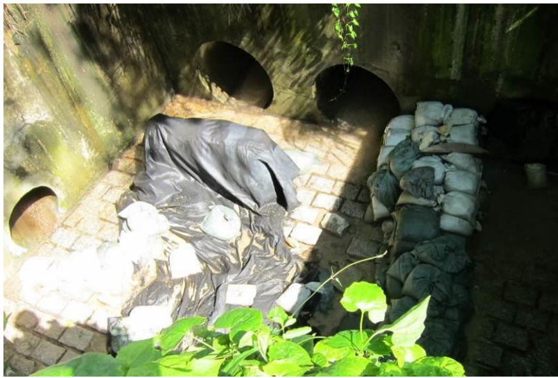
Stream B Outfall: Clean water is discharging.
