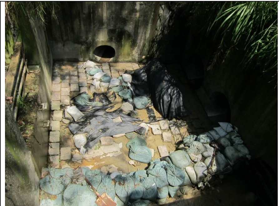
Stream B Outfall: Clean water is discharging.
