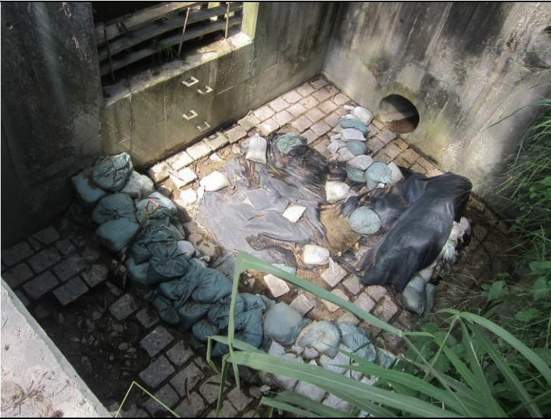
Stream B Outfall: Clean water is discharging.
