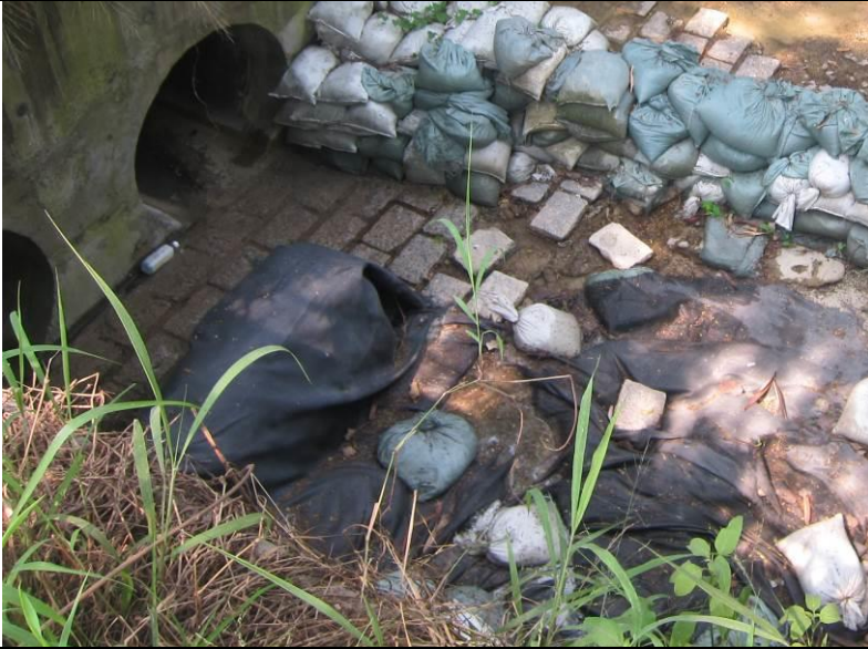
Stream B Outfall: Clean water is discharging.
