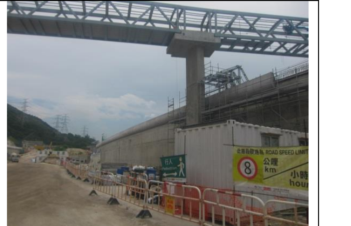
Photo 4 Set speed control at ~8km/hr for all vehicles using the haul road
