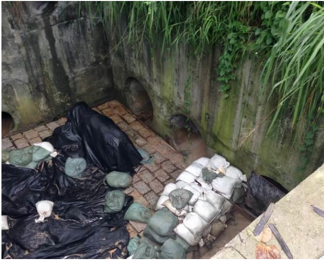
Stream B Outfall: Clean water is discharging.
