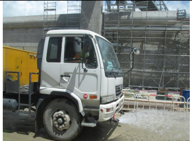
Photo 8 Watering of haul road by water truck to keep road surface wet was observed during the site inspection on 1 August 2017
