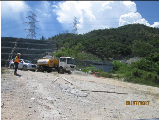
Photo 7 Watering of haul road by water truck to keep road surface wet was observed during the site inspection on 25 July 2017
