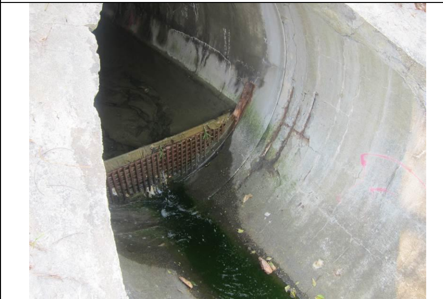
Outfall 1: Clean water is discharging.
