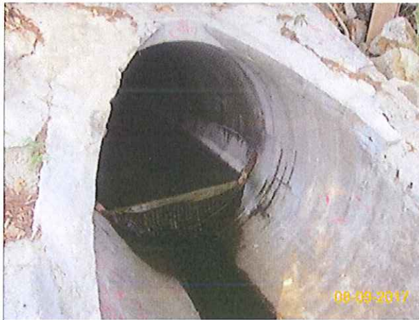
Item 7. Ensure no run-off into water body.
