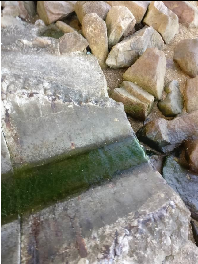
Outfall 1: Clean water is discharging.
