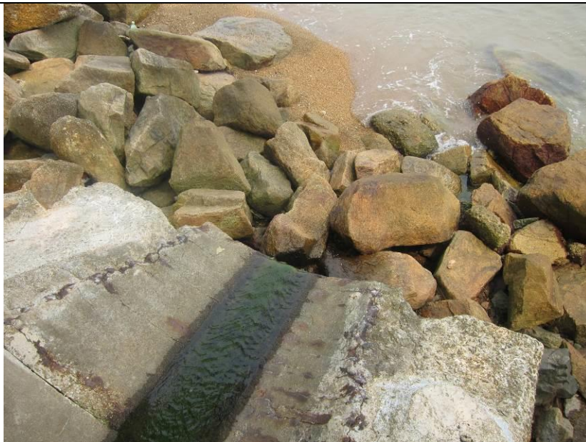
Outfall 1: Clean water is discharging.
