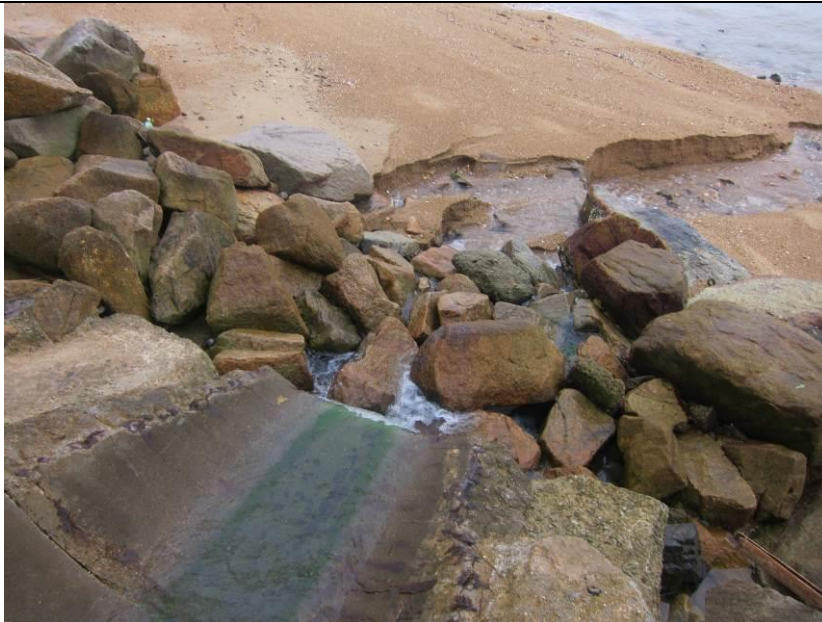
Outfall 1: Clean water is discharging.
