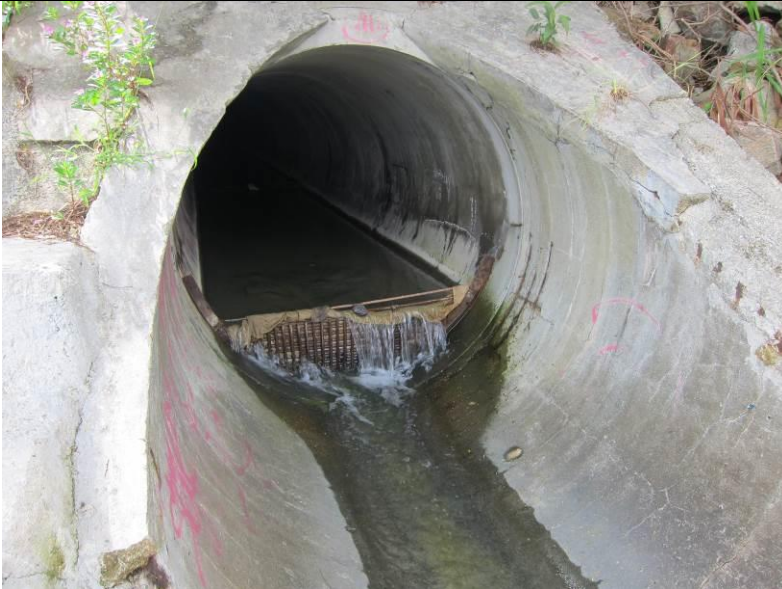
Outfall 1: Clean water is discharging.
