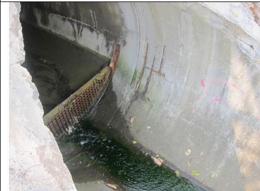
Outfall 1: Clean water is discharging.
