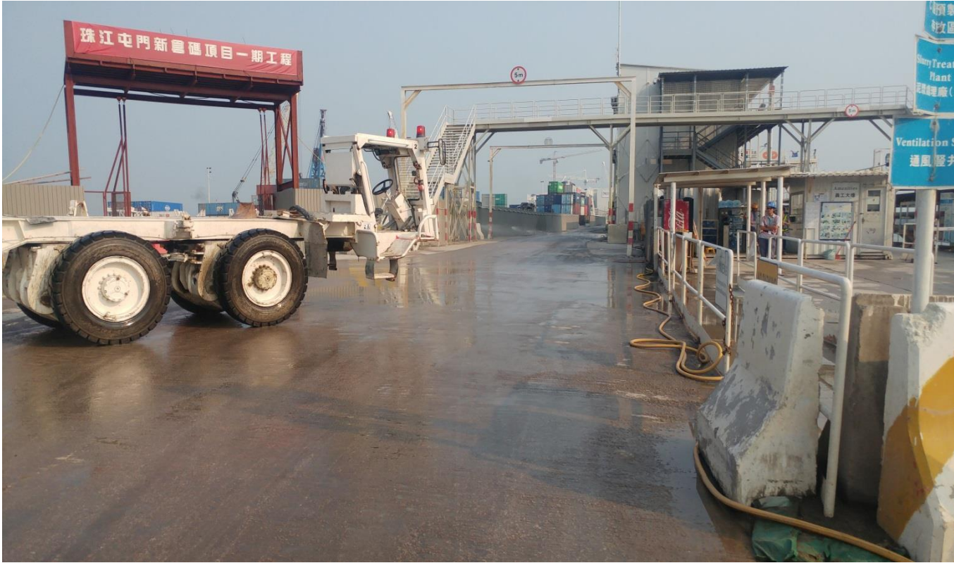
Water spraying was applied frequently during dry conditions. (Works Area Portion N-A)
