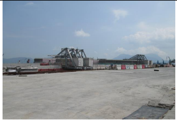
Photo 14 Housekeeping works at TD2 and most of the works area was hard paved.
