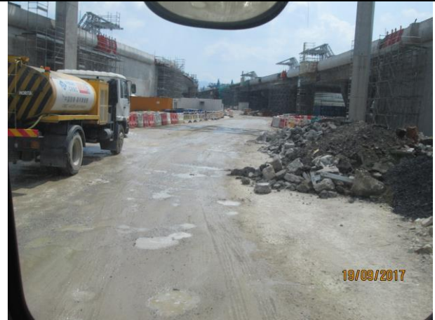
Photo 8 Watering of haul road by water truck to keep road surface wet was observed during the site inspection on 19 September 2017
