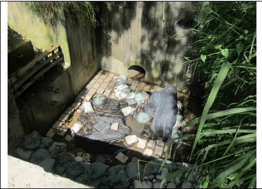
Stream B Outfall: Clean water is discharging.
