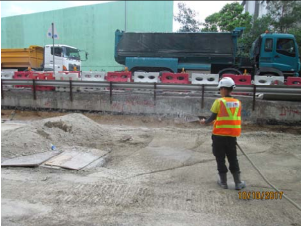
Photo 11 Water spraying was observed during the weekly inspection on 10 October 2017.
