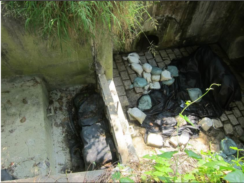
Stream B Outfall: Clean water is discharging.
