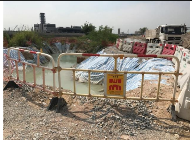
Photo 14 Exposed slope was covered with tarpaulin near TD2.
