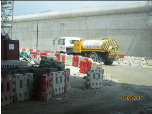
Photo 7 Watering of haul road by water truck to keep road surface wet was observed during the site inspection on 19 September 2017
