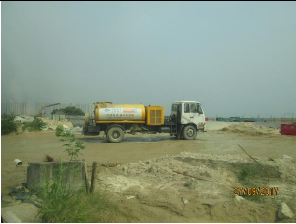
Photo 7 Watering of haul road by water truck to keep road surface wet was observed during the site inspection on 27 September 2017
