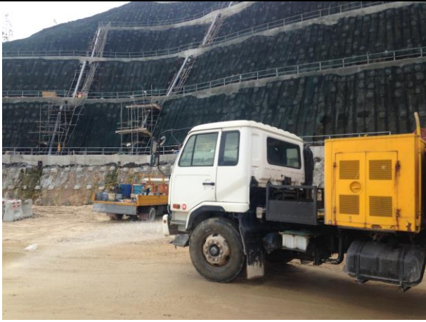
Photo 7 Watering of haul road by water truck to keep road surface wet was observed during the site inspection on 12 September 2017
