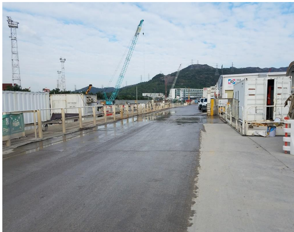
Water spraying was applied frequently during dry conditions. (Works Area Portion N-A)
