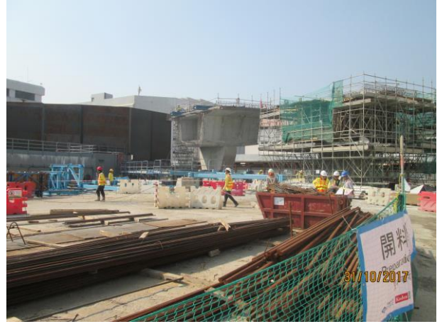
Photo 14 No dust emitted for the Portion F was observed during the site inspection on 31 October 2017 and the works area was clean and tidy
