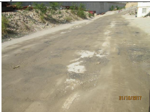
Photo 12 Watering of haul road by water truck to keep road surface wet was observed during the site inspection on 31 October 2017
