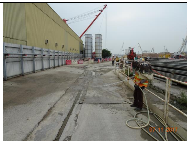
Photo 8 Watering of haul road to keep road surface wet was observed at Portion F during the site inspection on 7 November 2017
