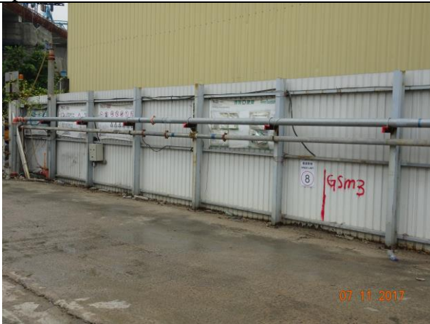
Photo 9 Set speed control at ~8km/hr for all vehicles using the haul road at Portion F
