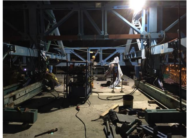
Finishing works at formtraveller during Night Time and limited light was used
