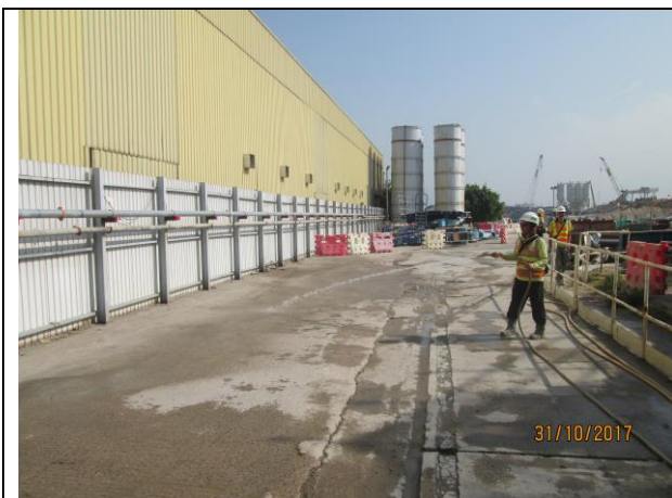
Photo 7 Watering of haul road to keep road surface wet was observed at Portion F during the site inspection on 31 October 2017
