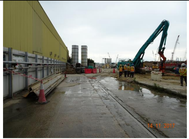
Photo 8 Watering of haul road to keep road surface wet was observed at Portion F during the site inspection on 14 November 2017
