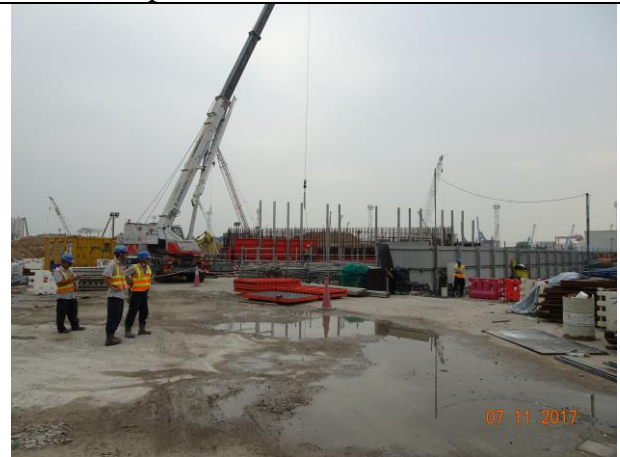
Photo 10 No dust emitted for the Portion F was observed during the site inspection on 7 November 2017 and the works area was clean and tidy
