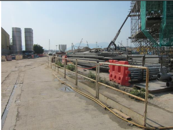
Photo 21 Construction of column at Portion F and most works area was hard paved.
