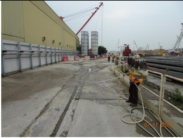
Photo 7 Watering of haul road to keep road surface wet was observed at Portion F during the site inspection on 7 November 2017
