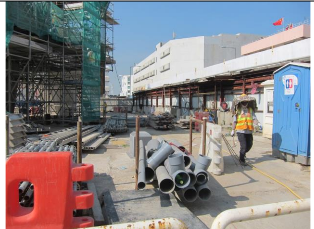
Photo 22 Construction of column at Portion F and most works area was hard paved.
