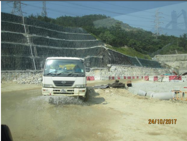
Photo 9 Watering of haul road by water truck to keep road surface wet was observed during the site inspection on 24 October 2017
