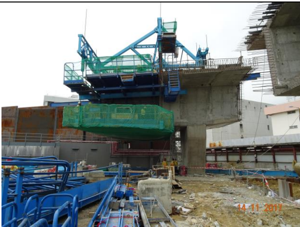
Photo 11 No dust emitted for the Portion F was observed during the site inspection on 14 November 2017 and the works area was clean and tidy
