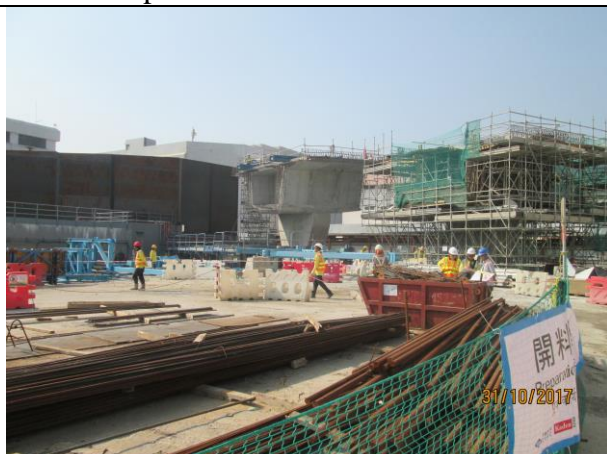
Photo 10 No dust emitted for the Portion F was observed during the site inspection on 31 October 2017 and the works area was clean and tidy
