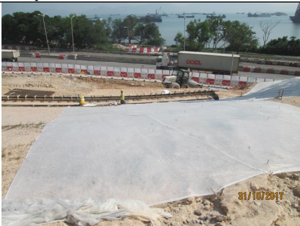
Photo 11 Photo taken of hydro seeding for the exposed sloop at slop 170 during the site inspection on 31 October 2017
