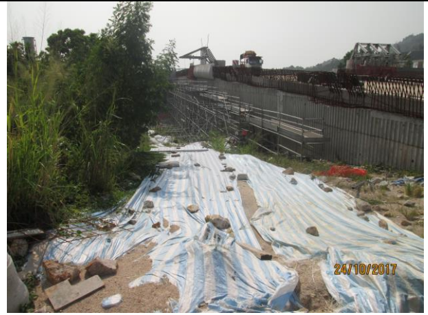
Photo 8 Covered part of the exposed slopes and stockpile by tarpaulin sheet was observed in the site inspection on 24 October 2017
