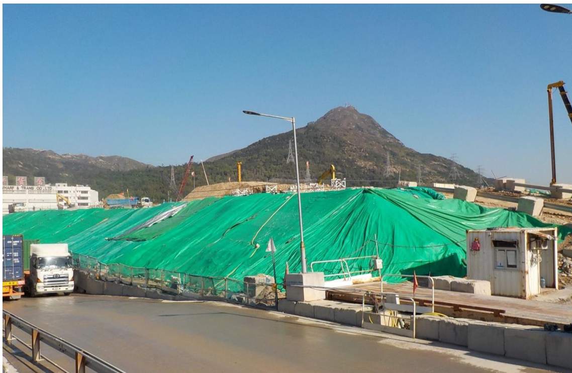
Exposed soil at Portion N-A was covered by tarpaulin sheets. (Works Area Portion N-A)
