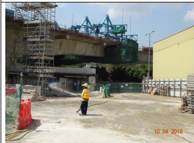
Photo 9 Site area keeping wet was observed at Portion F during the join site inspection on 10 April 2018
