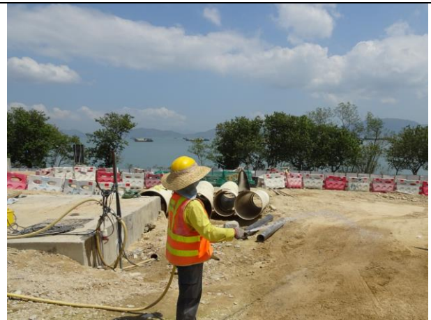
Photo 8 Site area keeping wet was observed at Portion H during the join site inspection on 10 April 2018
