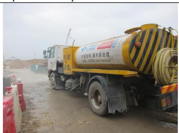
Photo 12 Watering of haul road and stockpile by water truck at Portion F
