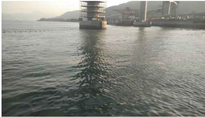
Photo 1 - Mid-Flood at SR4a on 3 January 2018
