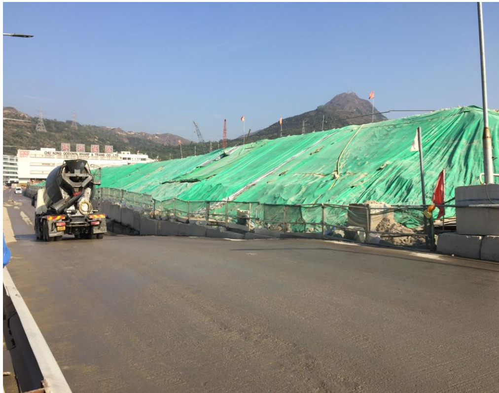
Exposed soil at Portion N-A was also covered by tarpaulin sheets. (Works Area Portion N-A)
