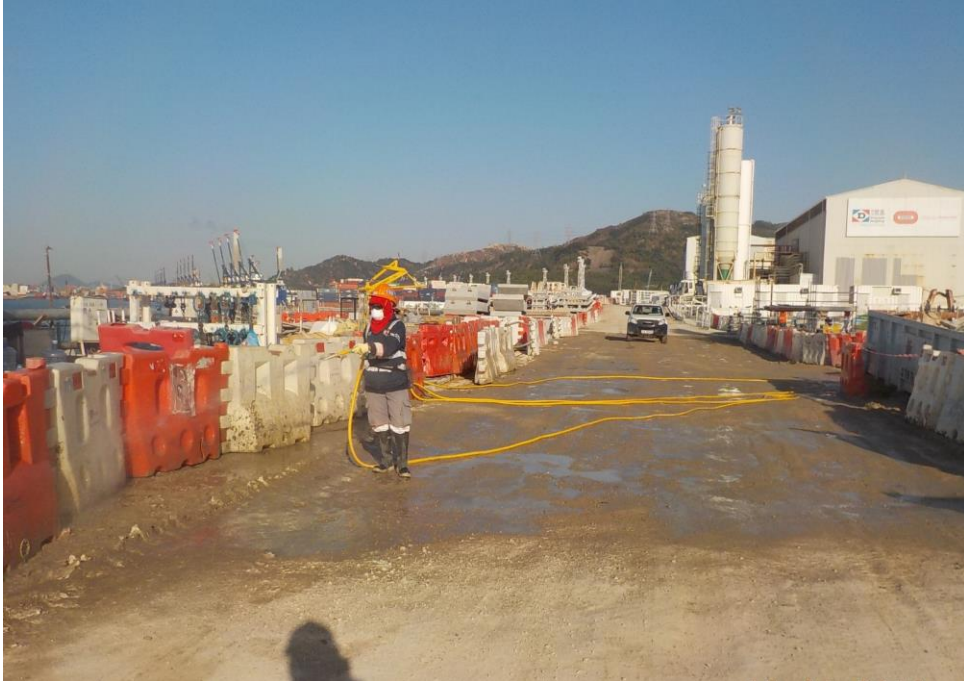
Water spraying was applied frequently during dry condition. (Works Area Portion N-B)
