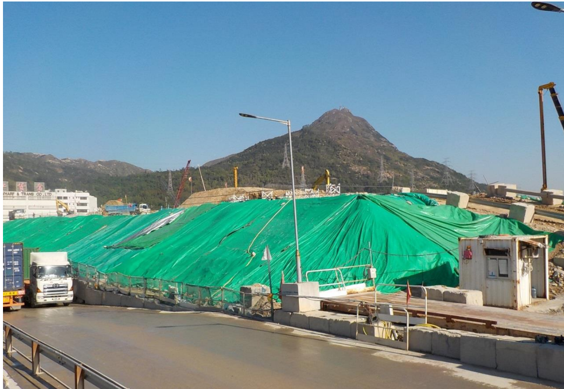
Exposed soil at Portion N-A was covered by tarpaulin sheets. (Works Area Portion N-A)
