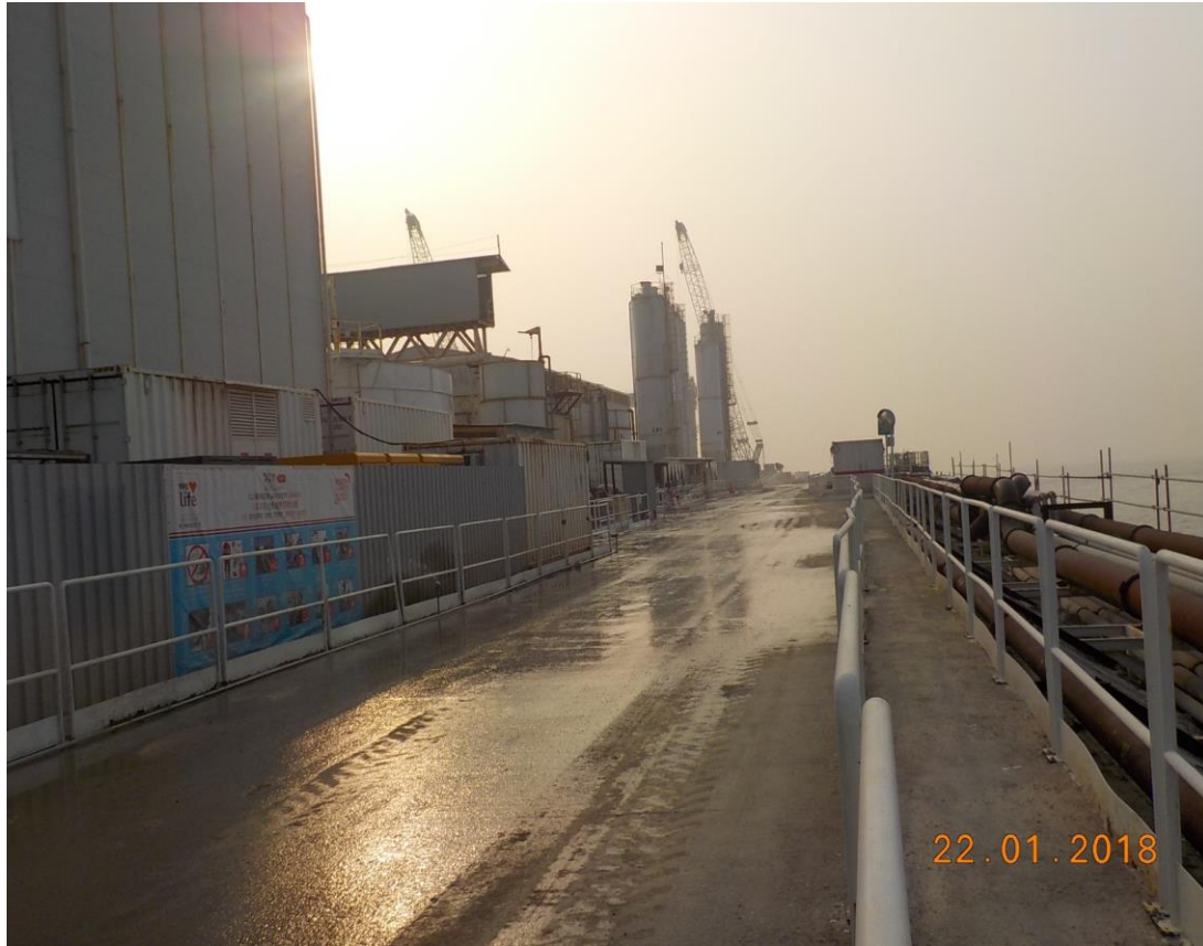
Water spraying was applied to prevent dust impact. (Works Area Portion N-B)
