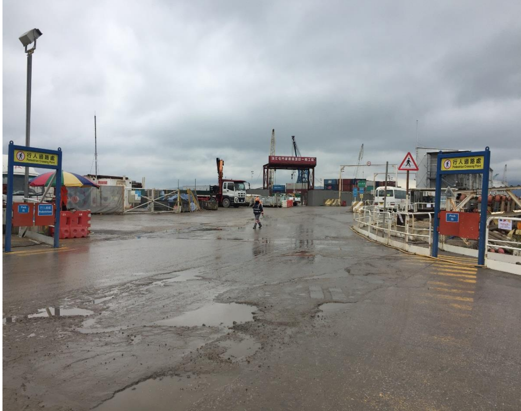
Water spraying was applied to prevent dust impact. (Works Area Portion N-A)
