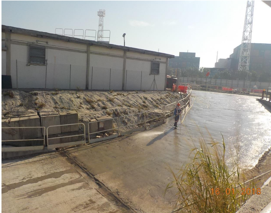
Water spraying was applied to prevent dust impact. (Works Area Portion N-A)
