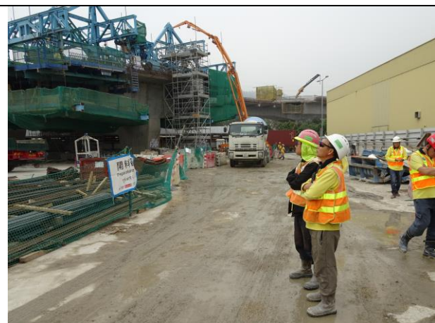
Photo 8 Site area keeping wet was observed at Portion F during the joint site inspection on 16 January 2018
