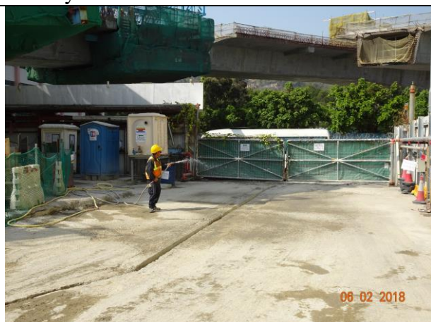
Photo 11 Watering of haul road to keep road surface wet was observed during the site inspection on 6 February 2018
