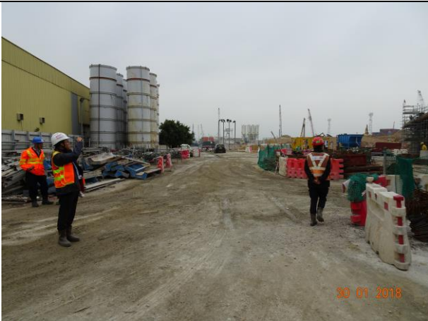
Keeping road surface wet to reduce dust impact at Portion F was observed during the weekly site inspection on 30 January 2018
