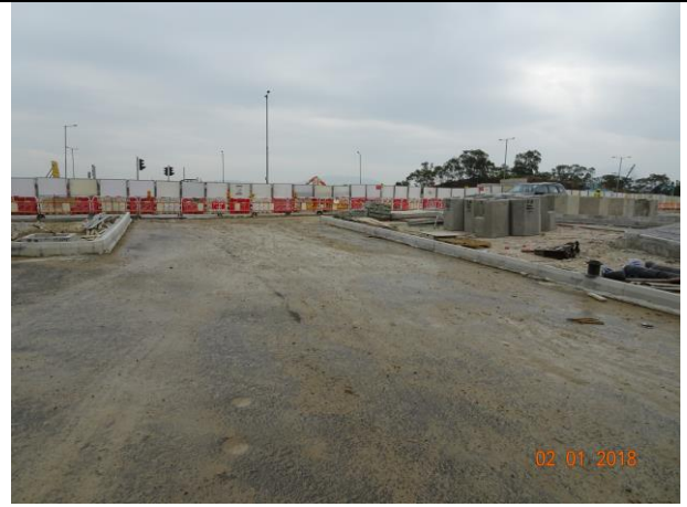
Photo 8 Site area keeping wet was observed at Portion H during the joint site inspection on 2 January 2018
