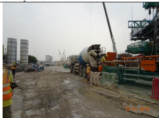
Photo 10 Site area keeping wet was observed at Portion F during the join site inspection on 23 January 2018
