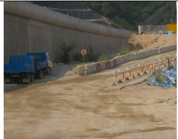
Photo 6 Set speed control at ~8km/hr for all vehicles using the haul road
