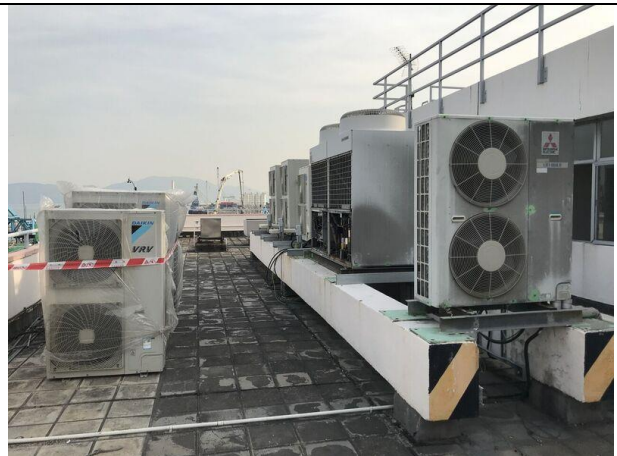
Photo 16 Photo taken on 6 February 2018 at the roof top of Pillar Point Fire Station
