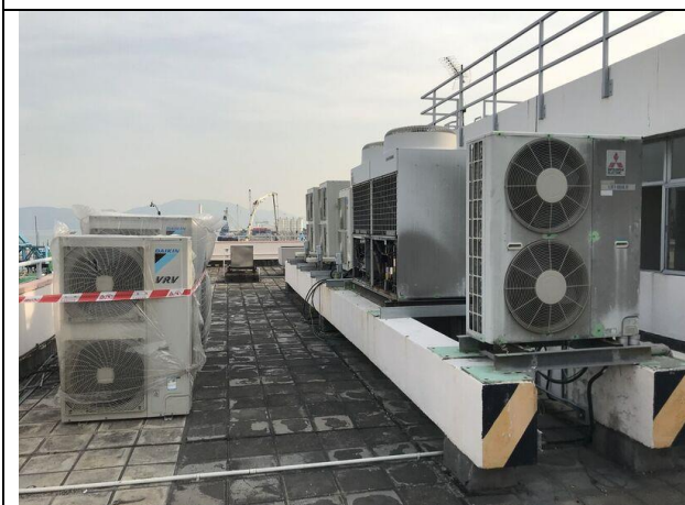
Photo 15 Photo taken on 6 February 2018 at the roof top of Pillar Point Fire Station
