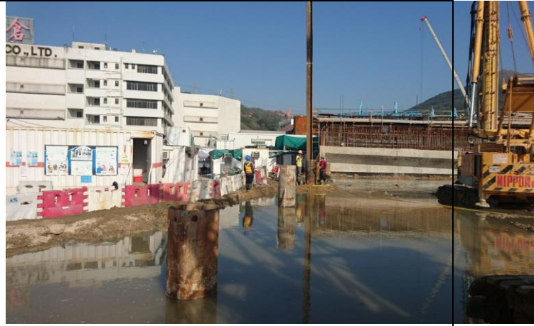
Photo 14 Construction of column at Portion F and most works area was keep wet.
