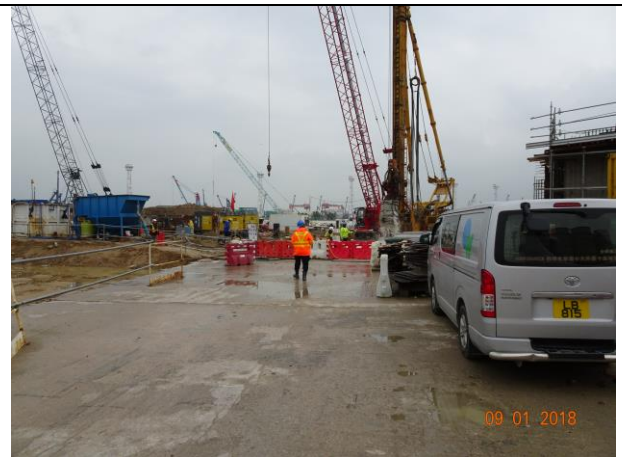
Keeping road surface wet to reduce dust impact at Portion F was observed during the weekly site inspection on 9 January 2018
