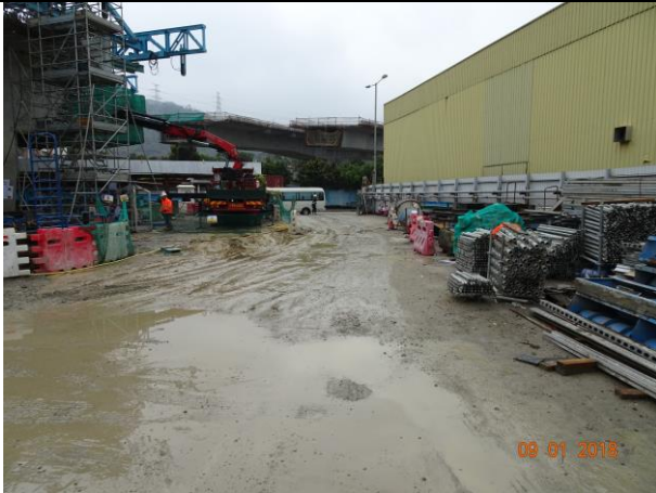
Photo 9 Site area keeping wet was observed at Portion F during the join site inspection on 9 January 2018
