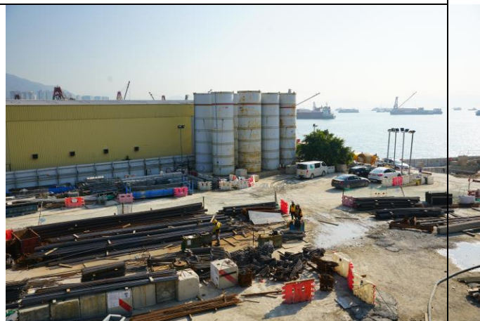
Photo 12 Construction of column at Portion F and most works area was keep wet.
