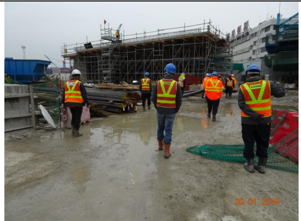
Keeping road surface wet to reduce dust impact at Portion F was observed during the weekly site inspection on 30 January 2018
