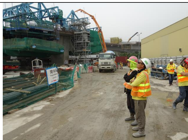
Photo 8 Site area keeping wet was observed at Portion F during the join site inspection on 16 January 2018
