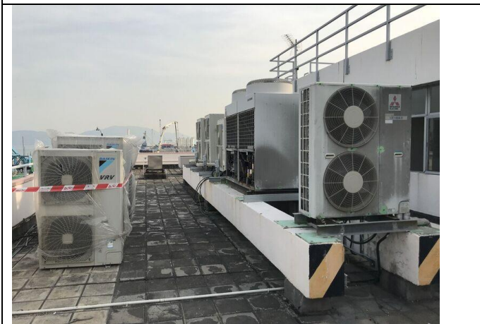
Photo 17 Photo taken on 6 February 2018 at the roof top of Pillar Point Fire Station
