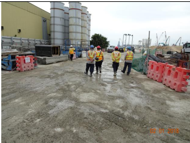
Watering of haul road to keep road surface wet was observed at Portion F during the weekly site inspection on 2 January 2018
