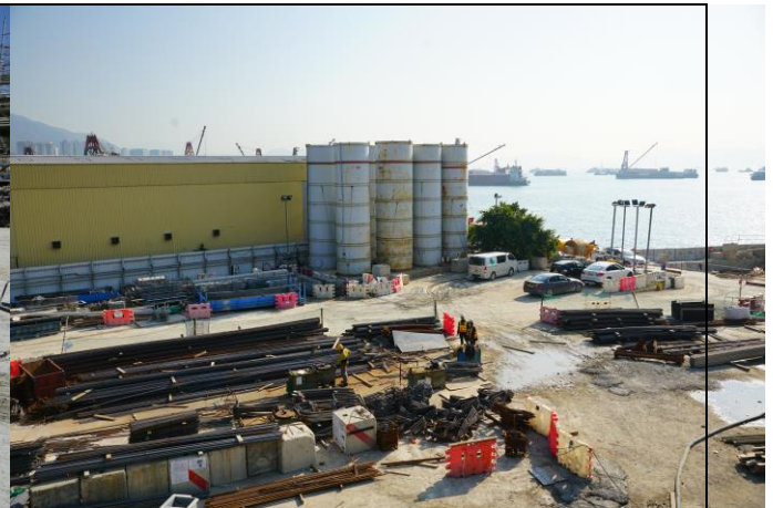
Photo 14 Construction of column at Portion F and most works area was keep wet.
