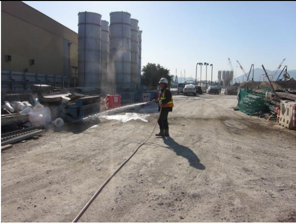
Watering of haul road to keep road surface wet was observed at Portion F during the weekly site inspection on 16 January 2018
