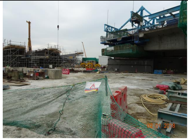
Photo 14 Construction of column at Portion F and most works area was hard paved.
