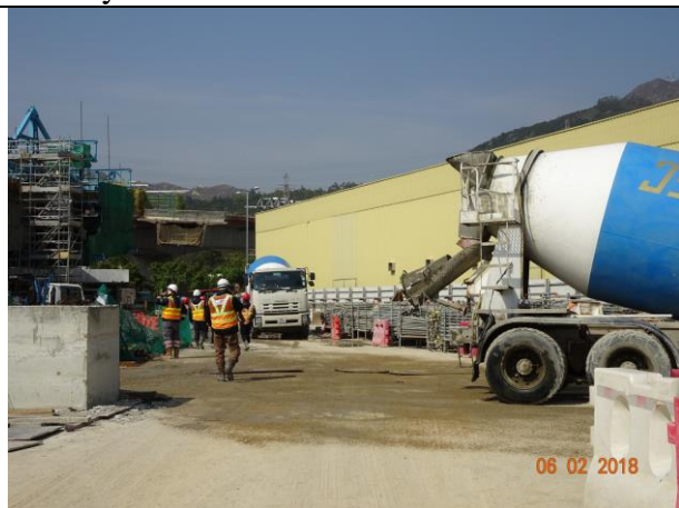
Photo 11 Site area keeping wet was observed at Portion F during the join site inspection on 6 February 2018
