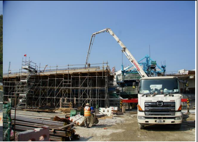
Photo 14 Construction of column at Portion F and most works area was keep wet.
