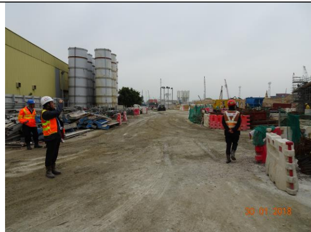
Photo 8 Site area keeping wet was observed at Portion F during the join site inspection on 30 January 2018
