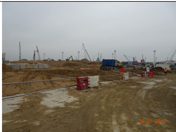
Photo 9 Site area keeping wet was observed at Portion F during the join site inspection on 30 January 2018
