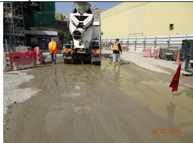
Photo 10 Site area keeping wet was observed at Portion F during the join site inspection on 6 February 2018
