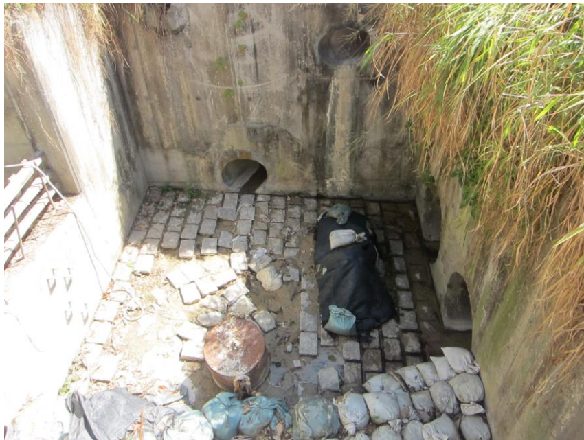
Stream B Outfall: No water is discharging.
