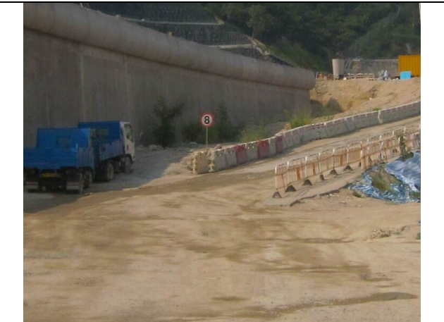
Photo 6 Set speed control at ~8km/hr for all vehicles using the haul road
