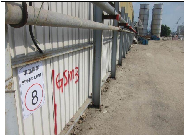
Photo 7 Set speed control at ~8km/hr for all vehicles using the haul road at Portion F
