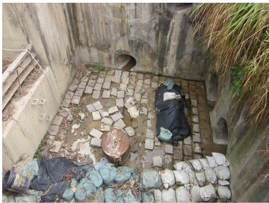
Stream B Outfall: No water is discharging.
