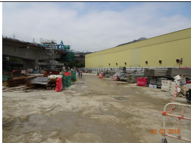
Photo 9 Site area keeping wet was observed at Portion F during the join site inspection on 20 March 2018
