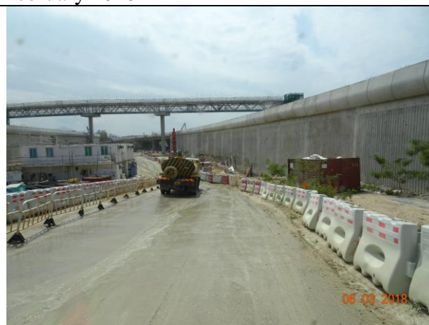
Photo 10 Water spraying by water truck was observed during the join site inspection on 6 March 2018
