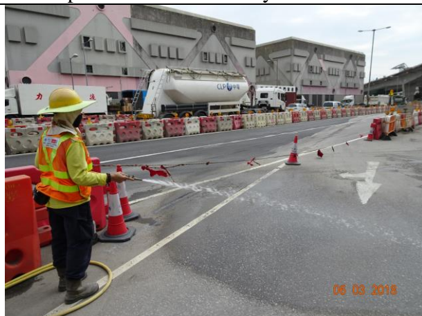
Photo 11 Site area keeping wet was observed at Lung Mun Road during the join site inspection on 6 March 2018
