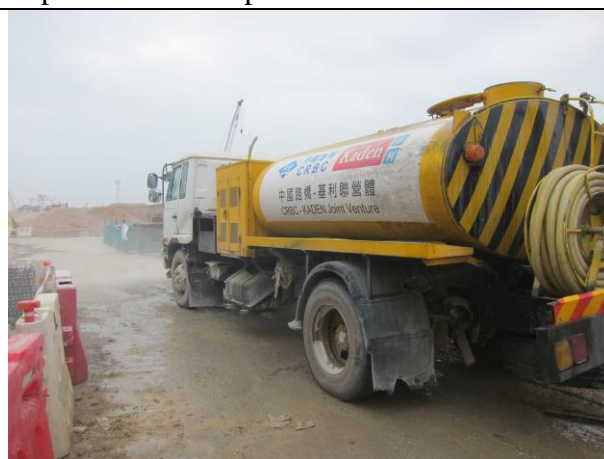
Photo 12 Watering of haul road and stockpile by water truck at Portion F
