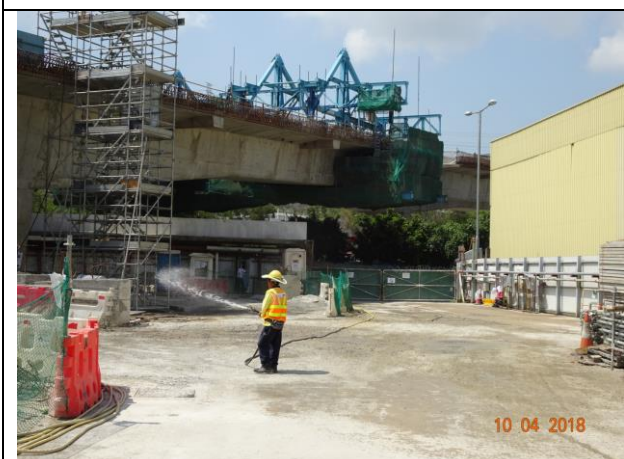
Photo 9 Site area keeping wet was observed at Portion F during the join site inspection on 10 April 2018
