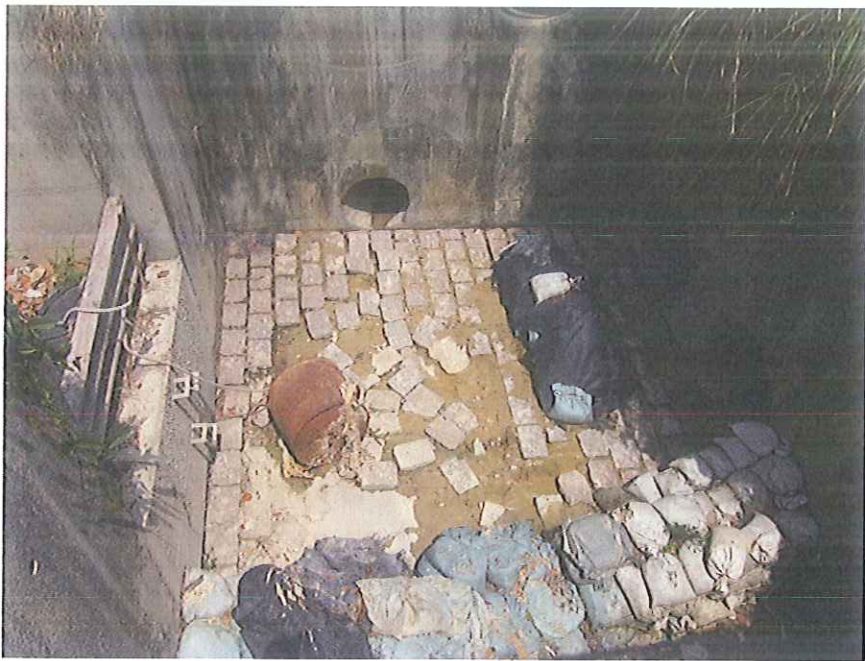
Stream B Outfall: No water is discharging.
