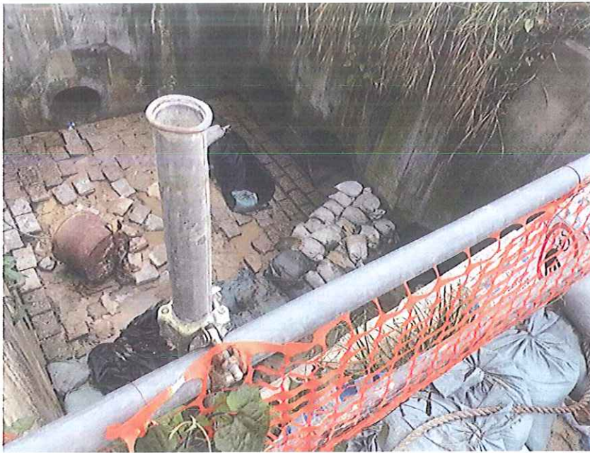
Stream B Outfall: No water is discharging.
