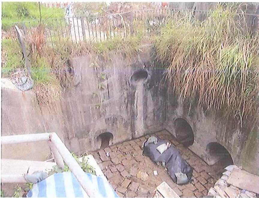
Stream B Outfall: No water is discharging.
