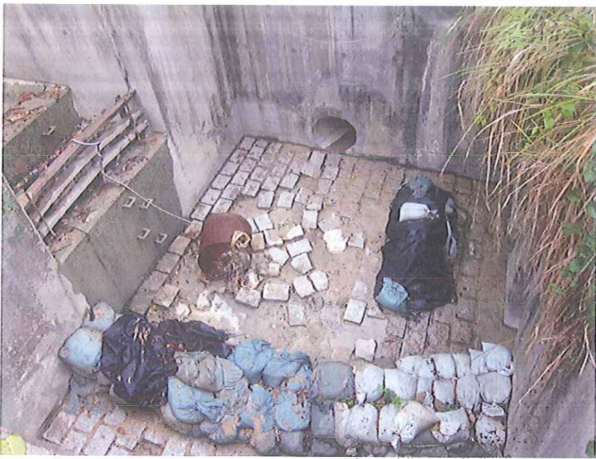
Stream B Outfall: No water is discharging.
