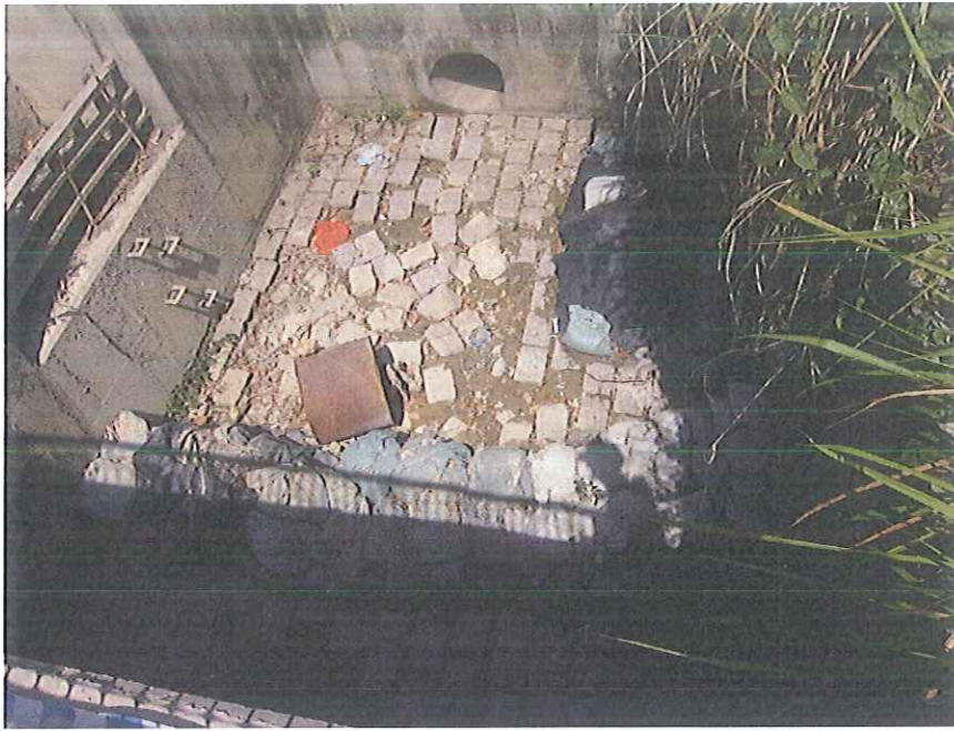
Stream B Outfall: No water is discharging.
