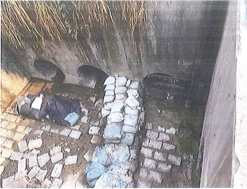
Stream B Outfall: No water is discharging.
