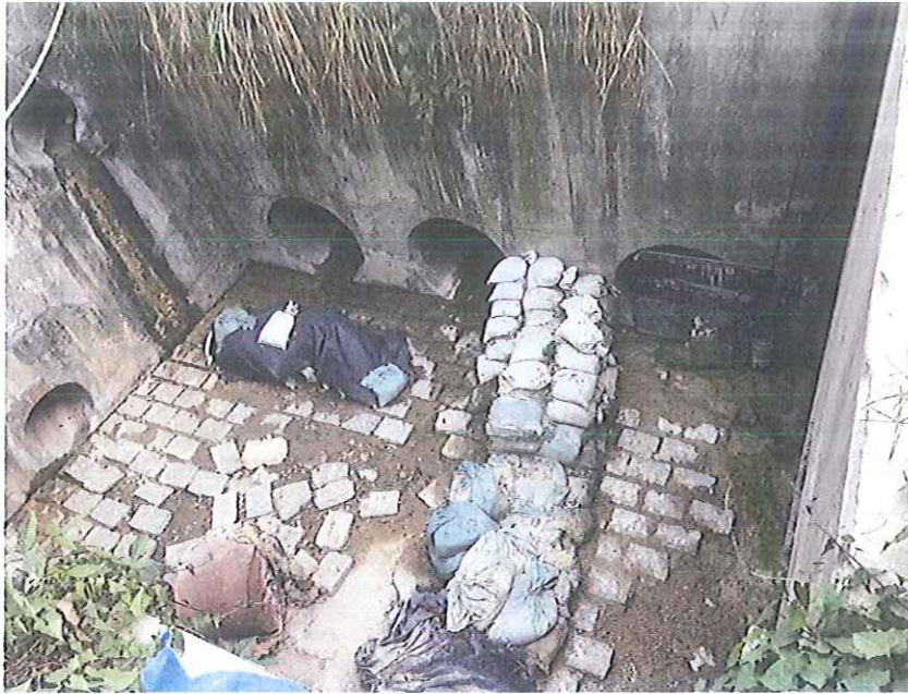
Stream B Outfall: No water is discharging.
