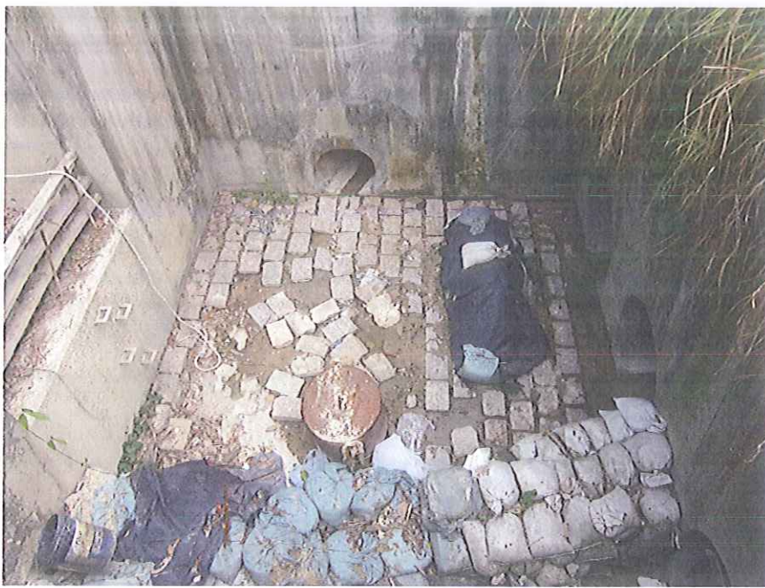
Stream B Outfall: No water is discharging.
