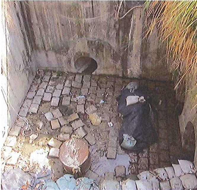
Stream B Outfall: No water is discharging.
