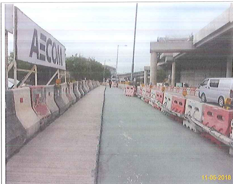
Item 5. Hoarding with panel around works area & Item 6. Temporary traffic management lighting.
