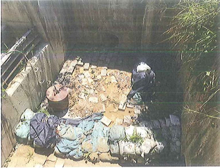
Stream B Outfall: No water is discharging.
