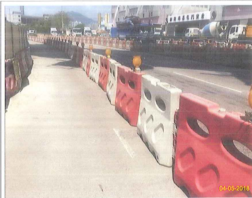
Item 5. Hoarding with panel around works area & Item 6. Temporary traffic management lighting.
