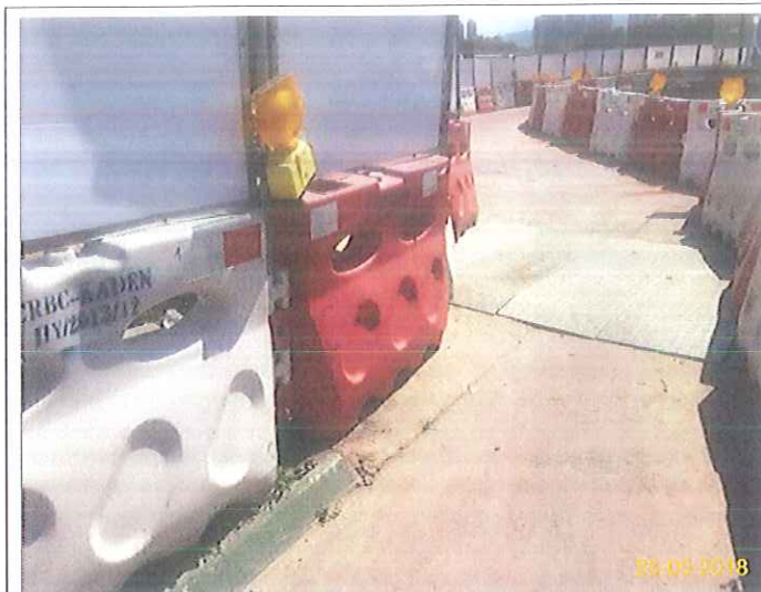
Item 5. Hoarding with panel around works area & Item 6. Temporary traffic management lighting.
