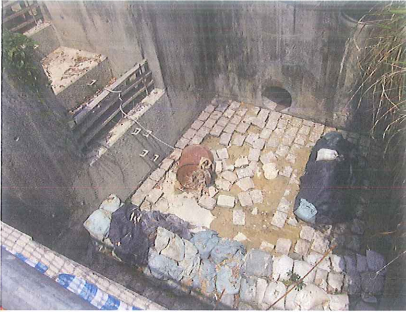
Stream B Outfall: No water is discharging.
