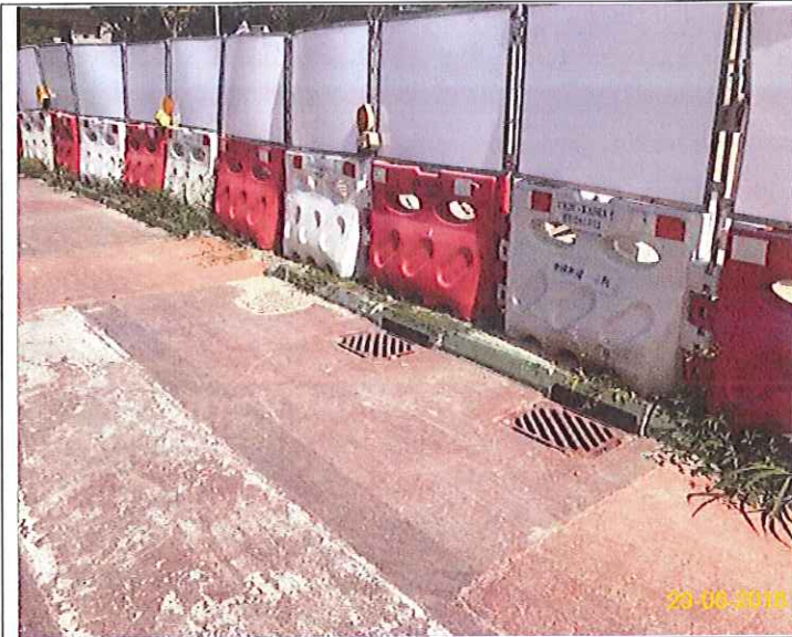
Item 5. Hoarding with panel around works area & Item 6. Temporary traffic management lighting.
