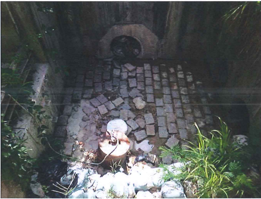
Stream B Outfall: Clean water is discharging.
