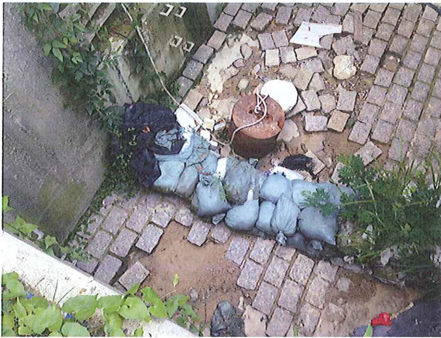
Stream B Outfall: Clean water is discharging.
