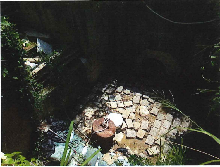
Stream B Outfall: Clean water is discharging.
