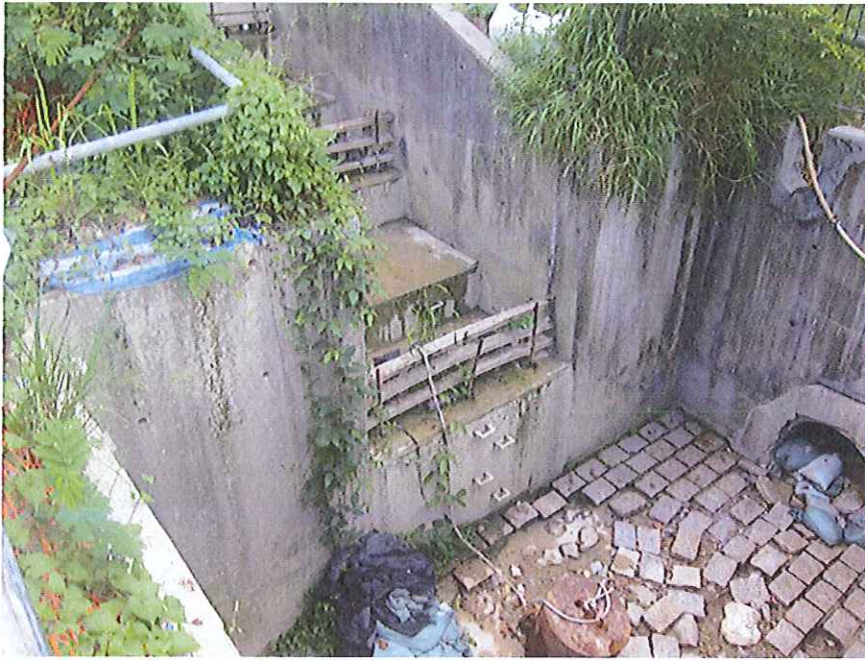
Stream B Outfall: Clean water is discharging.
