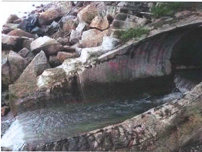
Outfall 1: Clean water is discharging.
