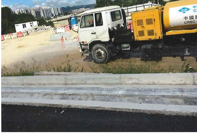
Photo 1 Watering of haul road by water truck to keep road surface wet
