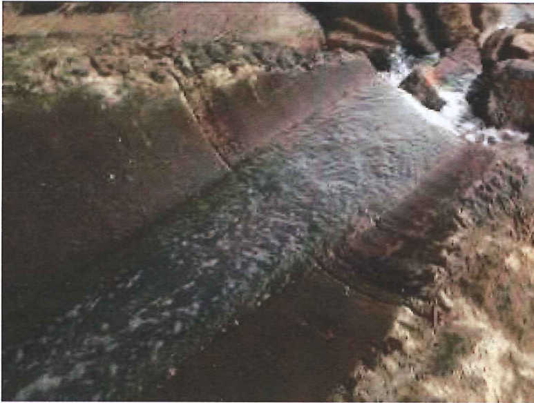
Outfall 1: Clean water is discharging.
