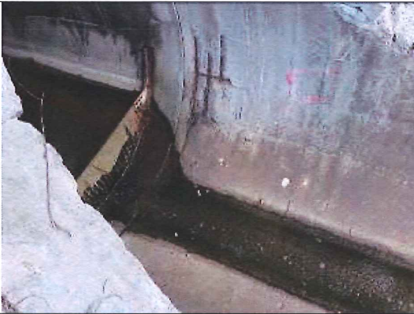
Outfall 1: Clean water is discharging.
