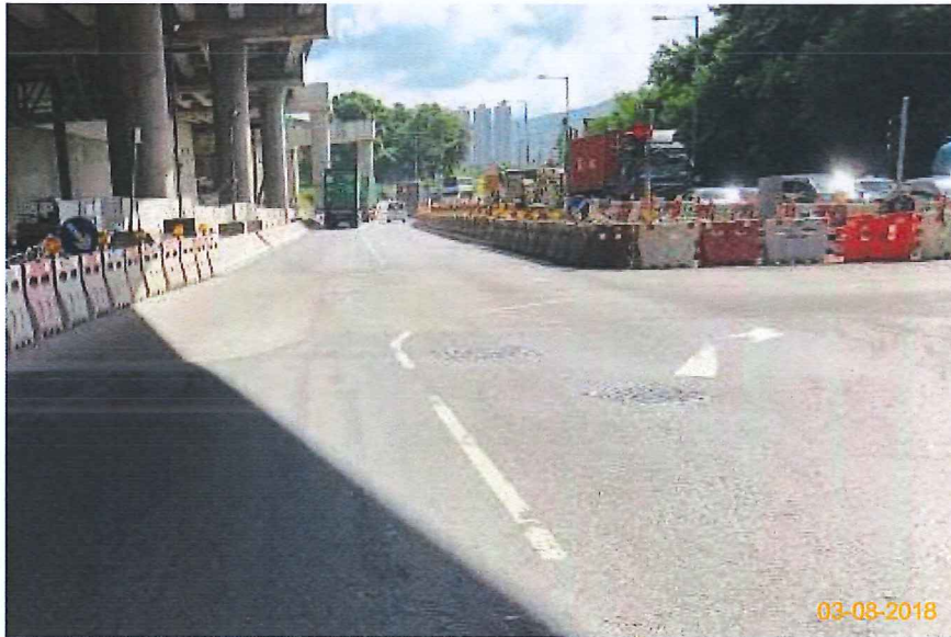
Item 5. Hoarding with panel around works area & Item 6. Temporary traffic management lighting.
