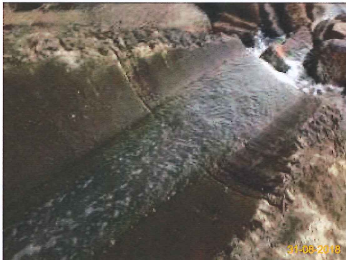
Item 7. Ensure no run-off into water body.(Outfall 1)
