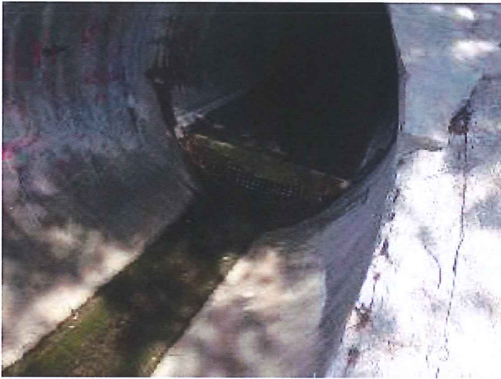
Outfall 1: Clean water is discharging.
