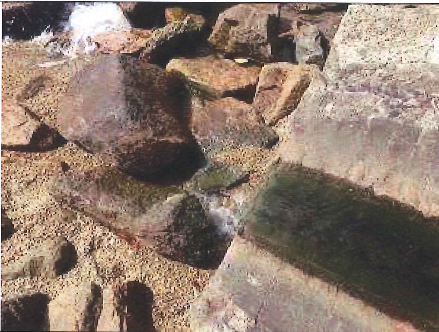
Outfall 1: Clean water is discharging.
