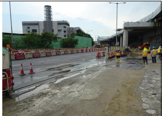
Photo 8 Dust mitigation measure was observed at Lung Mun Road during the joint site inspection on 28 August 2018.
