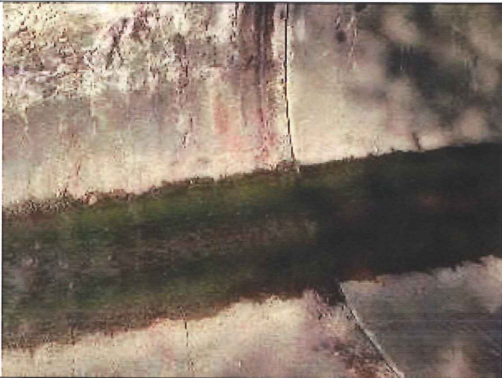
Outfall 1: Clean water is discharging.
