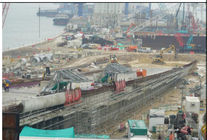
Photo 11 Stockpile stored at Portion F was backfilled and most of the site area was hard pave
