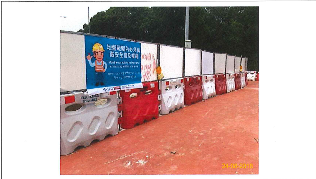
Item 5. Hoarding with panel around works area & Item 6. Temporary traffic management lighting.
