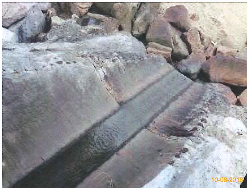
Item 7. Ensure no run-off into water body.(Outfall 1)
