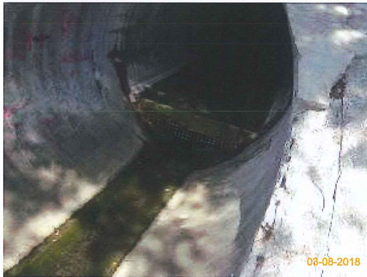
Item 7. Ensure no run-off into water body.(Outfall 1)
