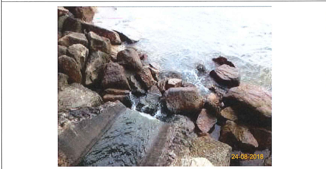
Item 7. Ensure no run-off into water body.(Outfall 1)
