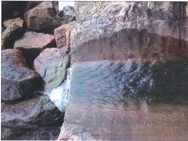
Outfall 1: Clean water is discharging.
