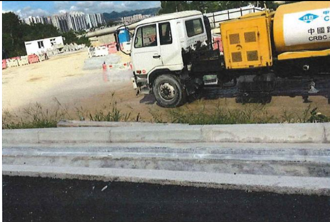
Photo 1 Watering of haul road by water truck to keep road surface wet
