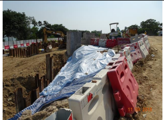
Photo 10 Dust mitigation measure was observed at exposed slope during the join site inspection on 11 September 2018.
