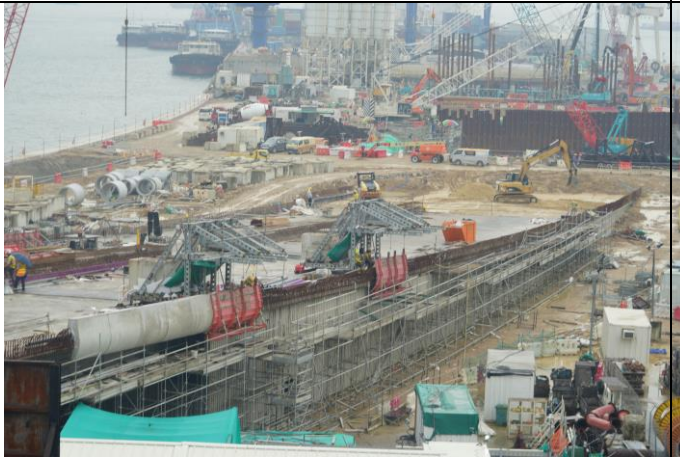
Photo 15 Stockpile stored at Portion F was backfilled and most of the site area was hard pave
