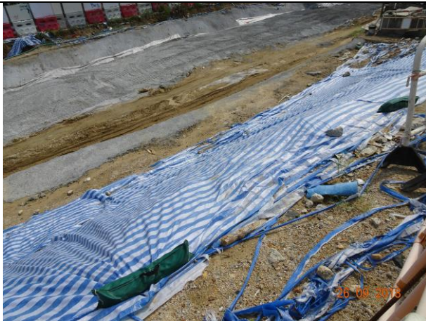
Photo 9 Dust mitigation measure was observed at exposed slope during the join site inspection on 26 September 2018.
