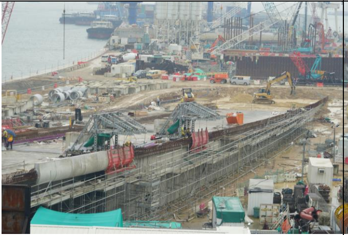
Photo 15 Stockpile stored at Portion F was backfilled and most of the site area was hard paved
