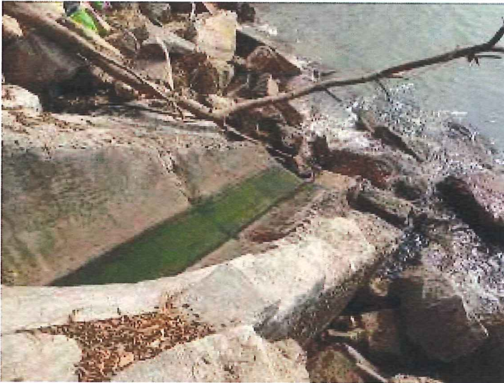
Outfall 1: Clean water is discharging.
