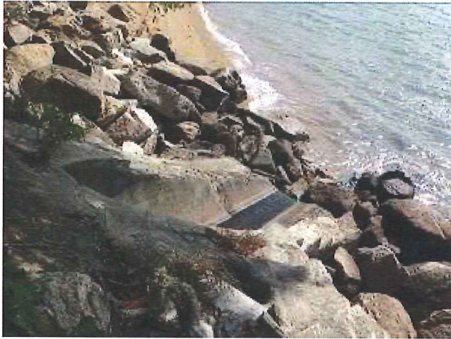
Outfall 1: Clean water is discharging.
