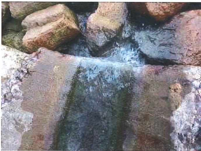
Outfall 1: Clean water is discharging.
