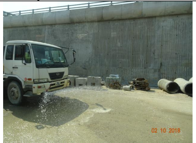
Photo 10 Dust mitigation measure was observed at site haul road during the join site inspection on 2 October 2018.
