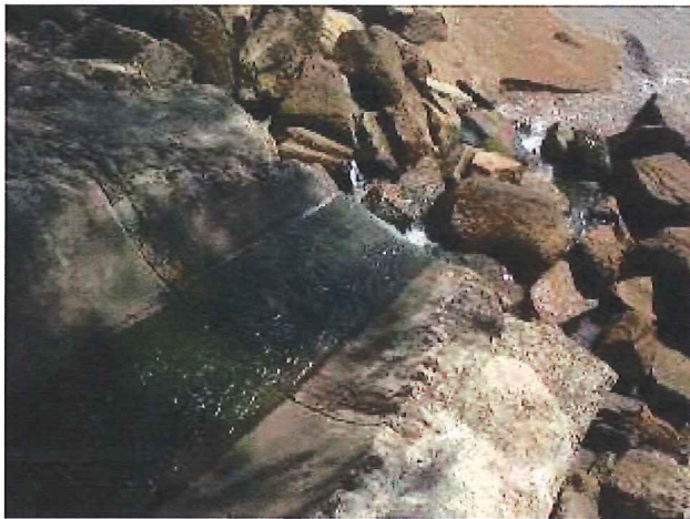
Outfall 1: Clean water is discharging.
