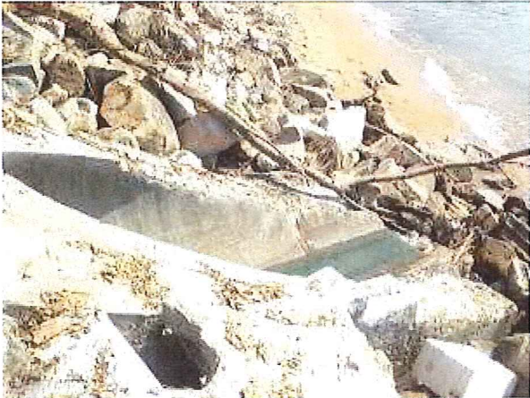
Outfall 1: Clean water is discharging.
