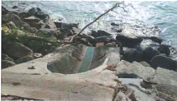
Outfall 1: Clean water is discharging.
