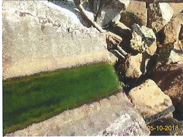
Item 7. Ensure no run-off into water body.(Outfall 1)
