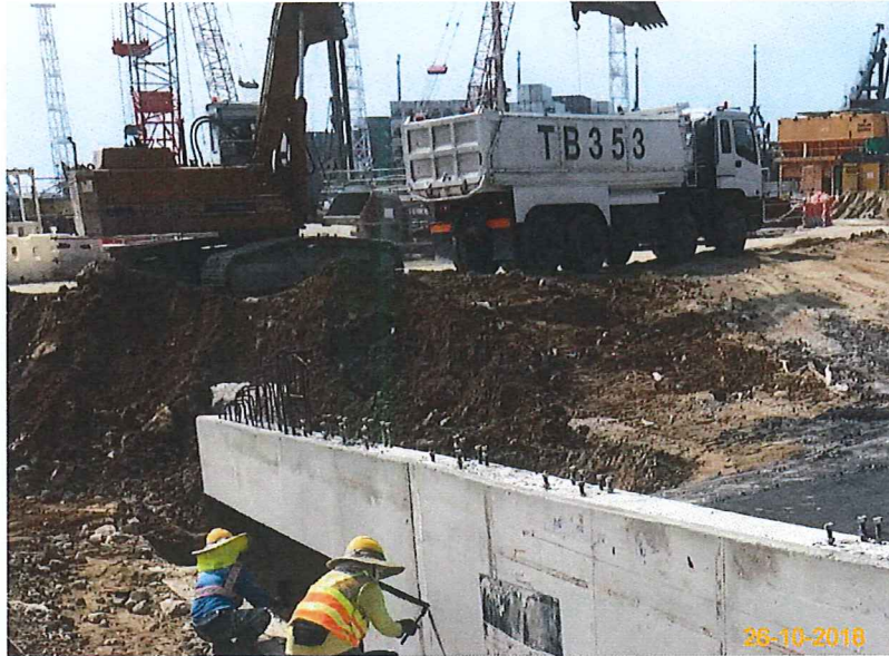
Item 4. Stockpile was removed from portion f.
