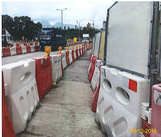
Item 5. Hoarding with panel around works area & Item 6. Temporary traffic management lighting.
