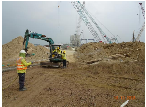
Photo 10 Dust mitigation measure was observed for the stockpile and site haul road at portion F during the join site inspection on 10 October 2018.
