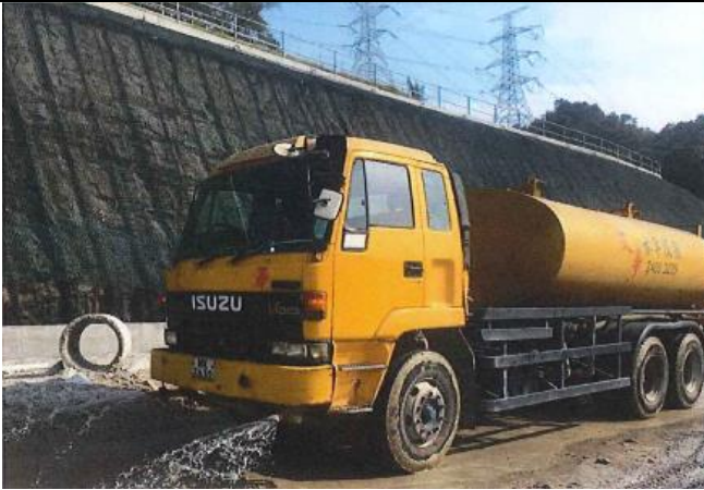
Photo 1 Watering of haul road by water truck to keep road surface wet
