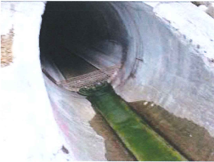
Outfall 1: Clean water is discharging.
