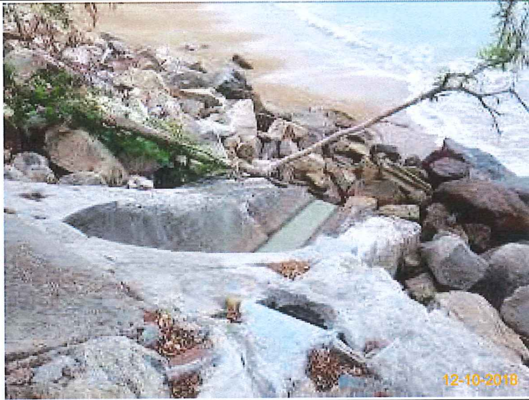
Item 7. Ensure no run-off into water body.(Outfall 1)
