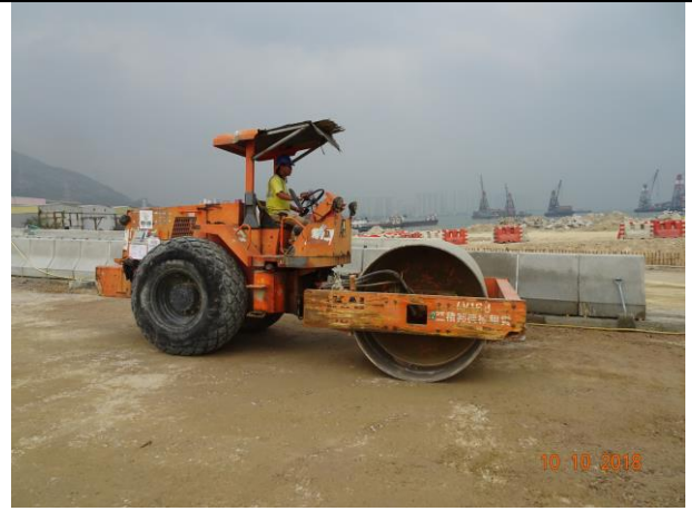
Photo 8 Compact the exposed surface was observed at Portion F to reduce dust impact was observed during the join site inspection on 10 October 2018.
