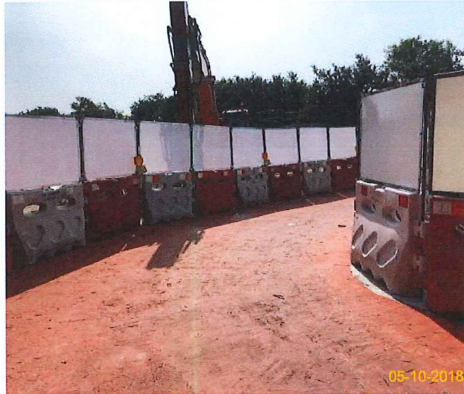
Item 5. Hoarding with panel around works area & Item 6. Temporary traffic management lighting.
