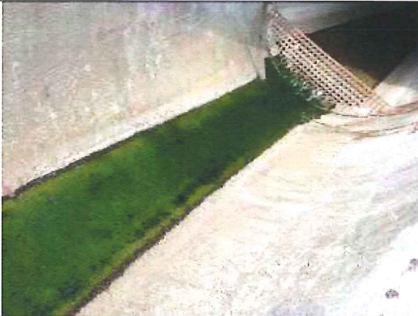
Outfall 1: Clean water is discharging.
