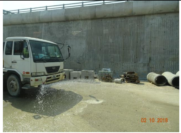
Photo 8 Dust mitigation measure was observed at site haul road during the join site inspection on 2 October 2018.
