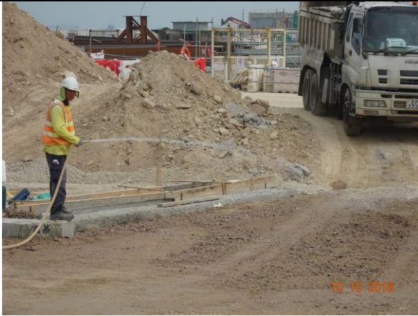
Photo 9 Dust mitigation measure was observed for the stockpile and site haul road at portion F during the join site inspection on 10 October 2018.
