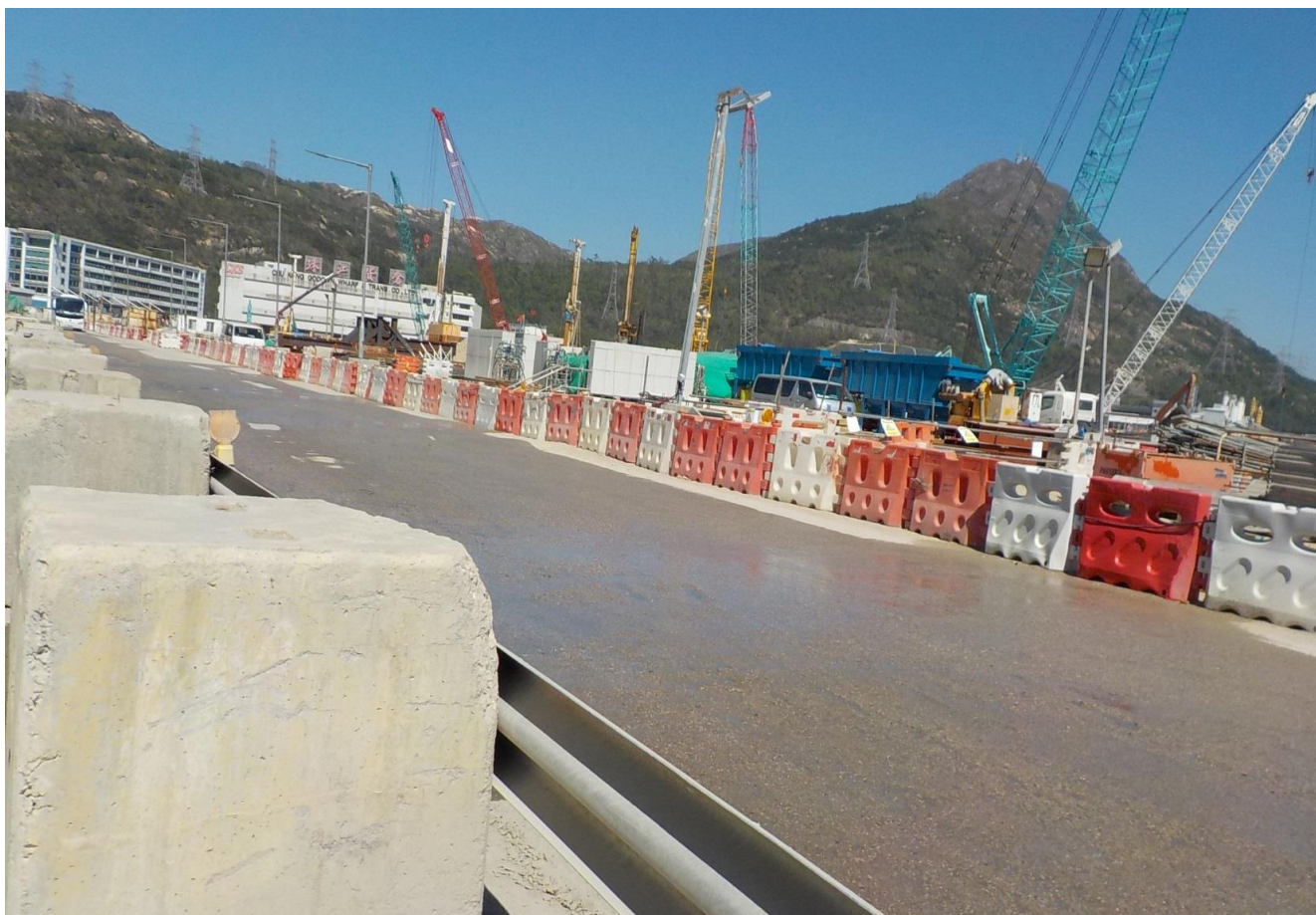
Water spraying was applied on the main haul road. (Works Area Portion N-A)
