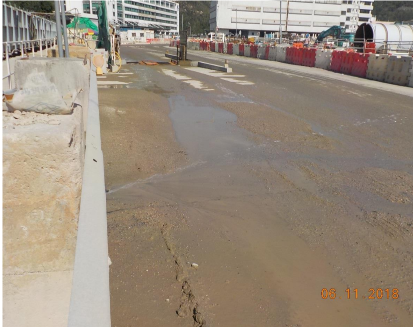
Water spraying was applied on the main haul road. (Works Area Portion N-A)
