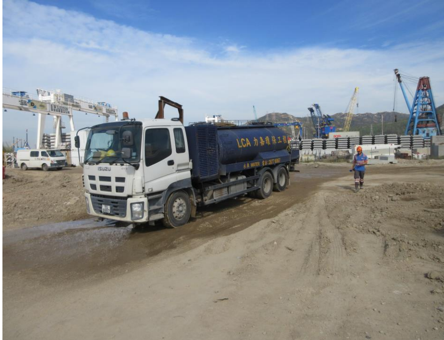
Water spraying was applied on the main haul road. (Works Area Portion N-A)
