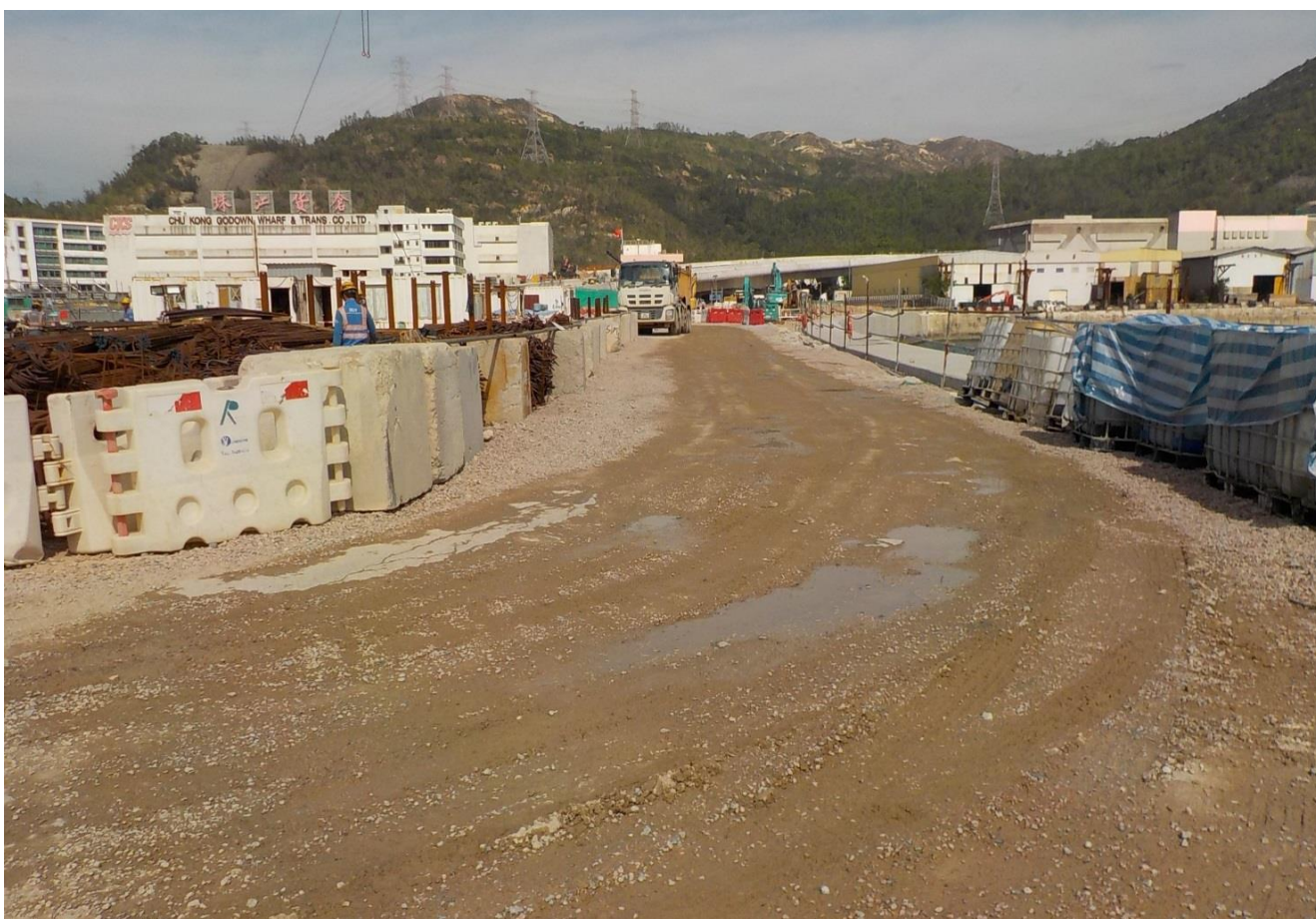
Water spraying was applied on the main haul road. (Works Area Portion N-A)
