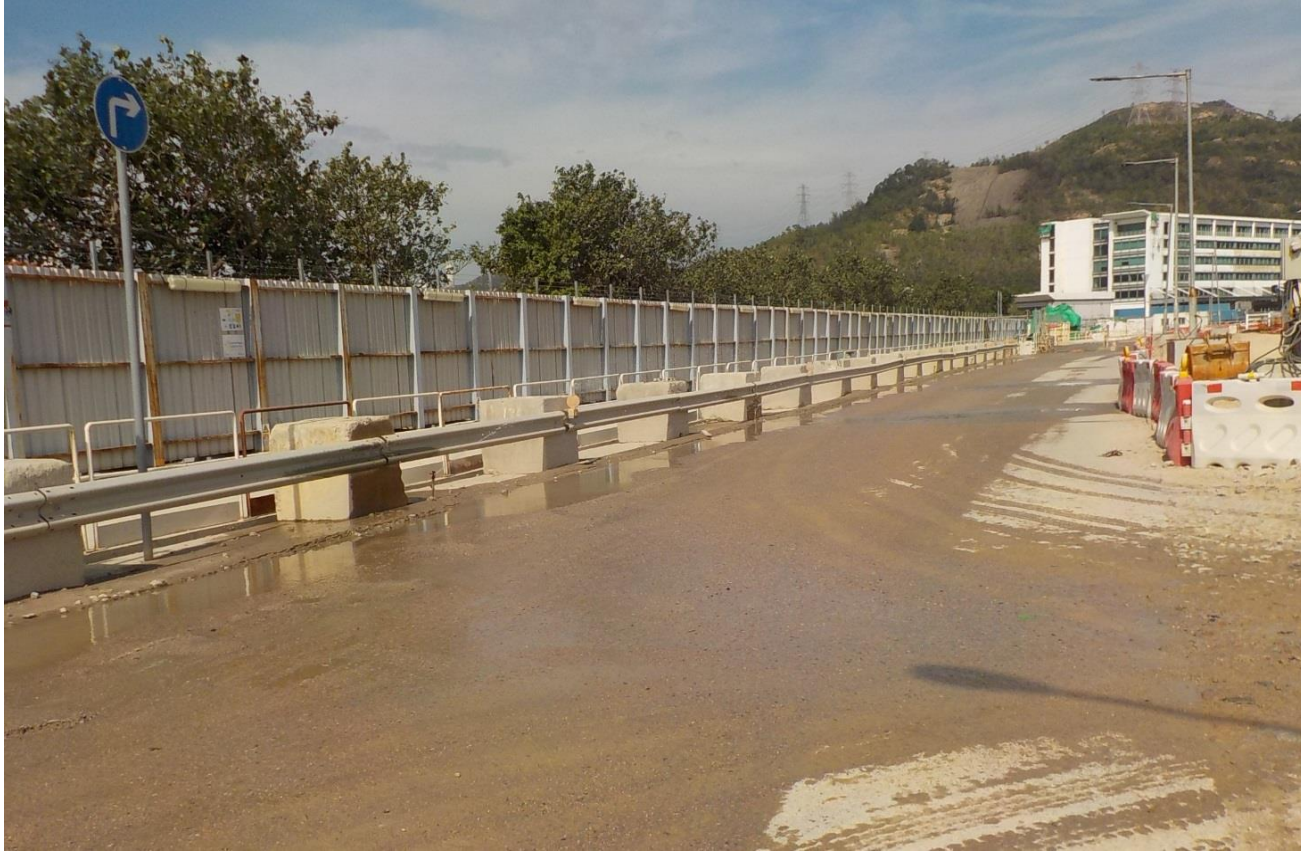
Water spraying was applied on the main haul road. (Works Area Portion N-A)
