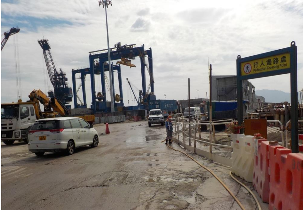
Water spraying was applied on the main haul road. (Works Area Portion N-A)
