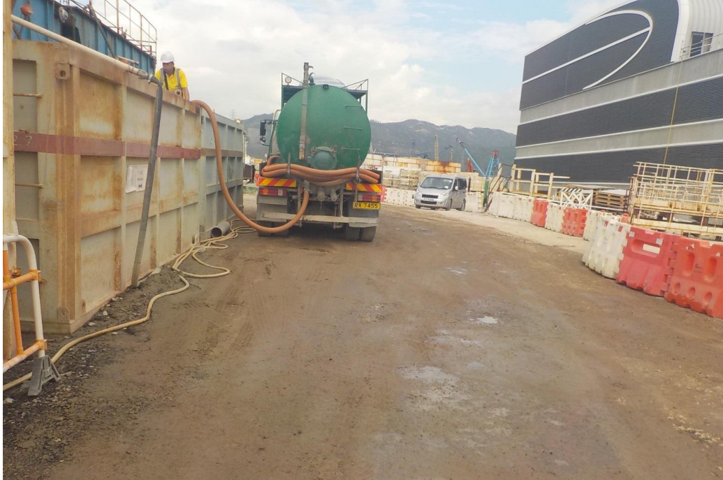
Water truck was used for dust control during surcharge removal. (Works Area Portion N-C)
