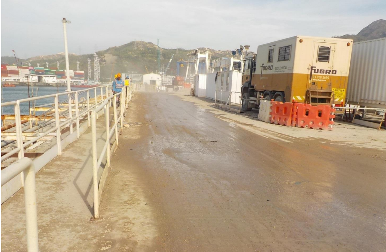
Water spraying was applied on the main haul road. (Works Area Portion N-C)
