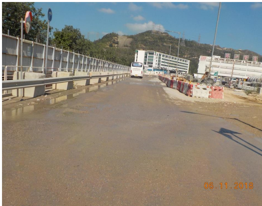
Water spraying was applied on the main haul road. (Works Area Portion N-A)
