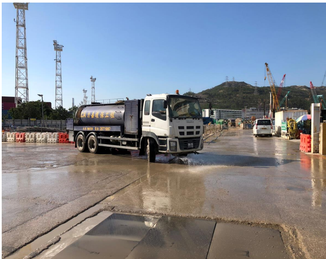
Water spraying was applied on the main haul road. (Works Area Portion N-A)
