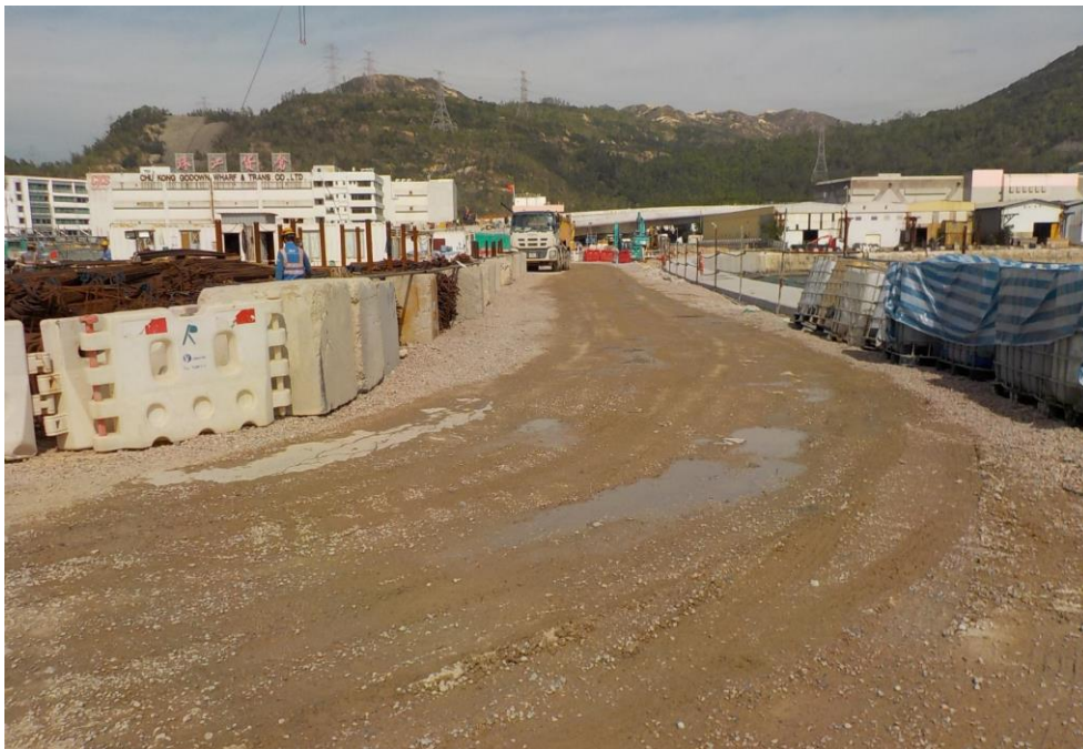
Water spraying was applied on the main haul road. (Works Area Portion N-A)
