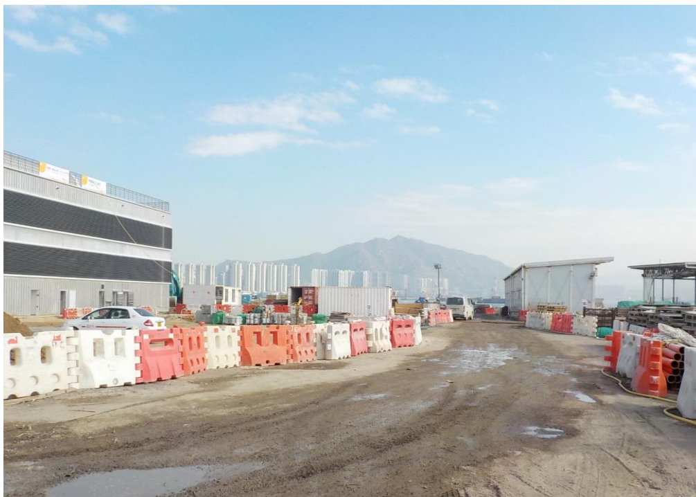
Water spraying was applied on the main haul road. (Works Area Portion N-C)
