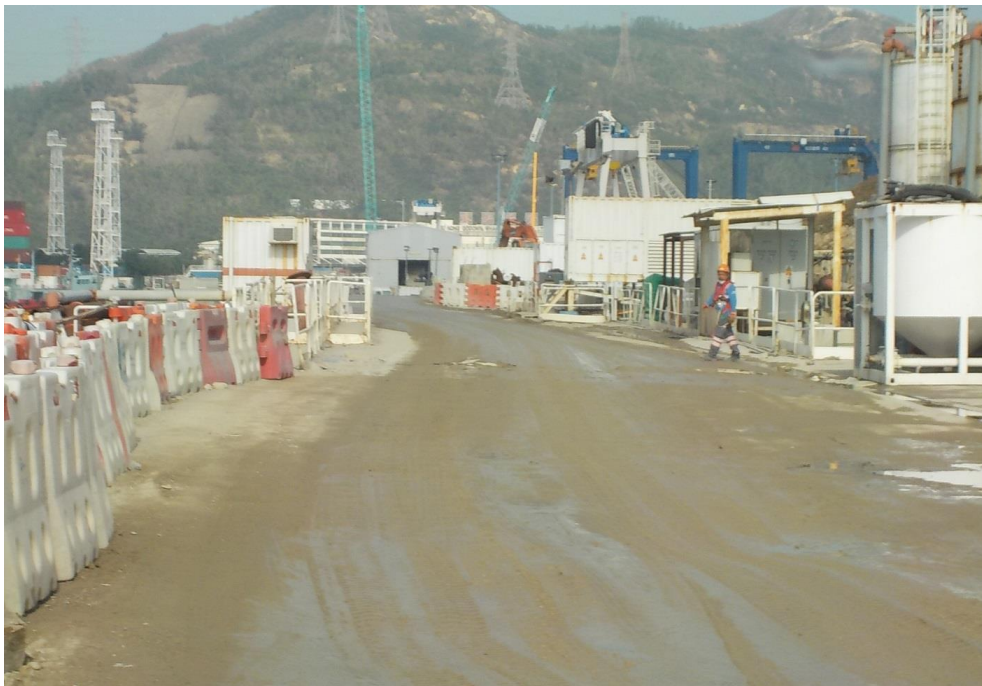
Water spraying was applied on the main haul road. (Works Area Portion N-C)
