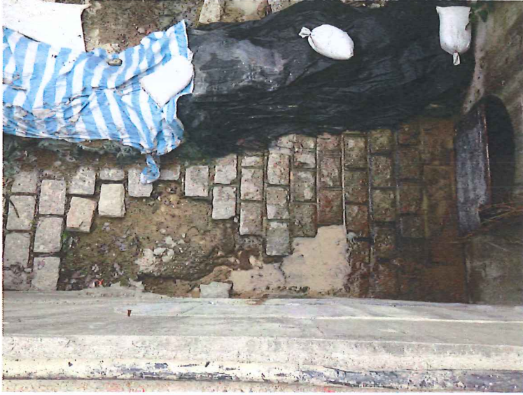
Stream B Outfall: No water is discharging.
