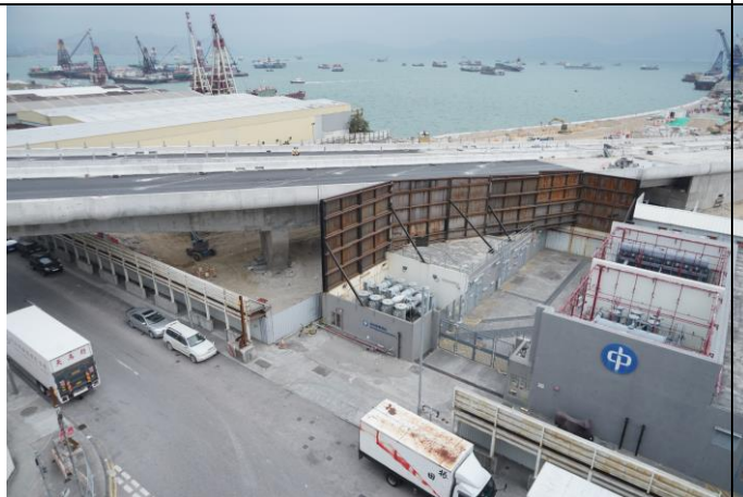
Photo 11 Stockpile stored at Portion F was backfilled and most of the site area was hard paved
