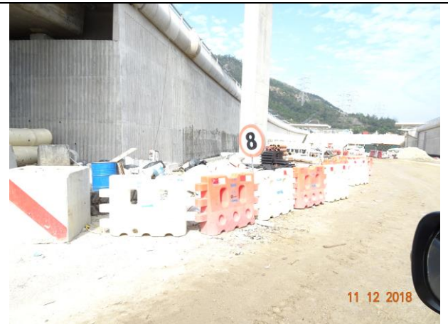
Photo 6 Set speed control at ~8km/hr for all vehicles using the haul road
