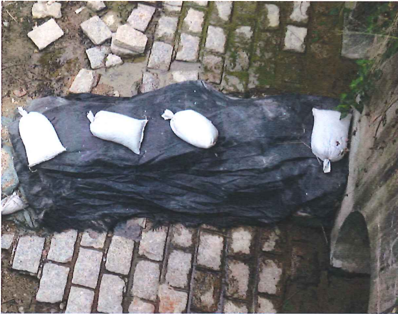
Stream B Outfall: No water is discharging.
