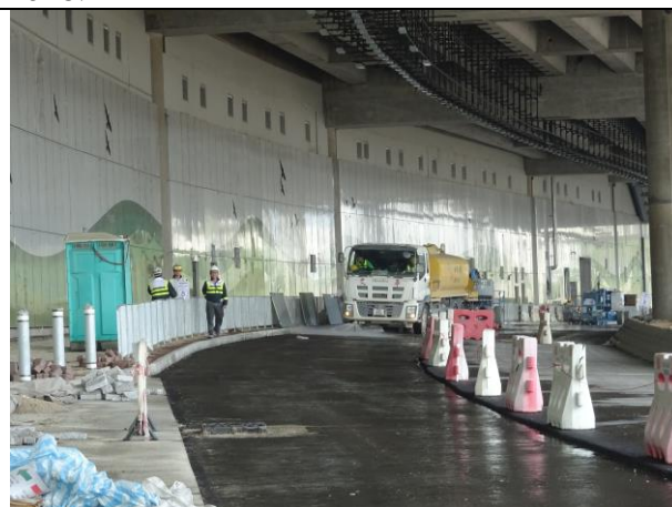
Photo 10 Dust mitigation measure was observed at site haul road during the joint site inspection on 18 December 2018.
