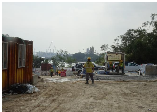
Photo 9 Dust mitigation measure was observed at site haul road during the joint site inspection on 18 December 2018.
