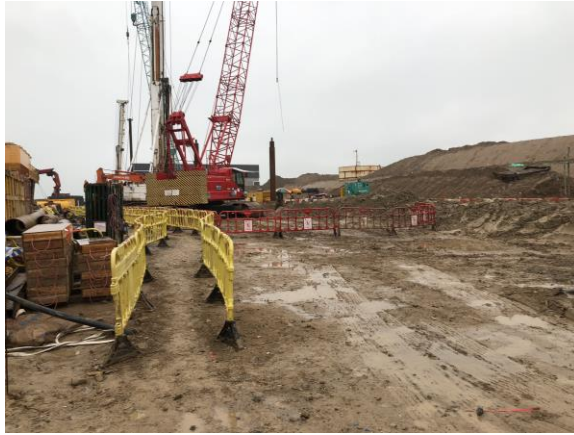
Photo 1 - Watering of unpaved roads at works area near Fire Services Department Building to maintain a wet condition (7 December 2018)
