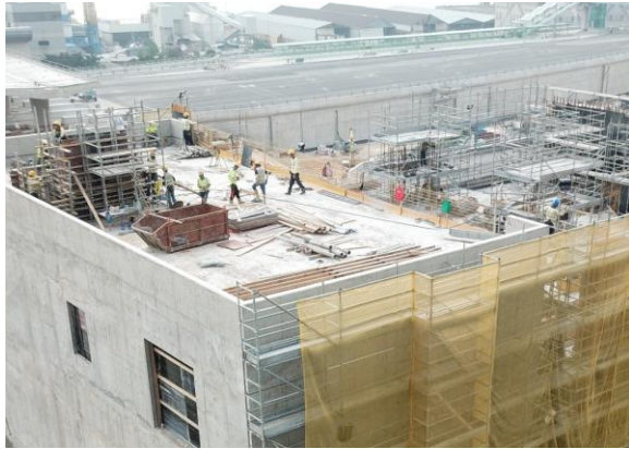
Photo 1 - Falsework, rebar fixing and formwork conducted at works area of Toll Control Building
