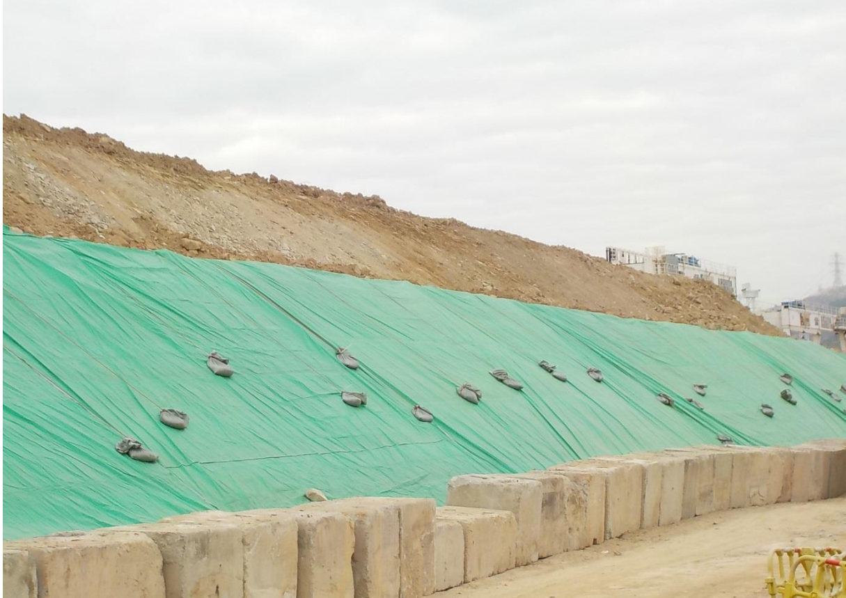
Exposed soil are covered by tarpaulin sheets to prevent dust. (Works Area Portion N-C)
