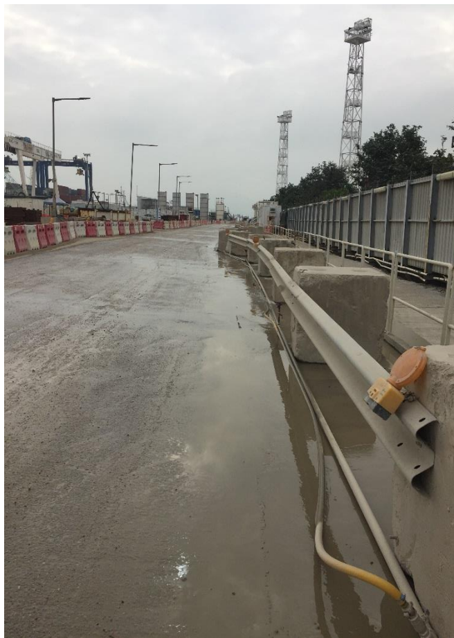
Water spraying was applied on the main haul road. (Works Area Portion N-A)
