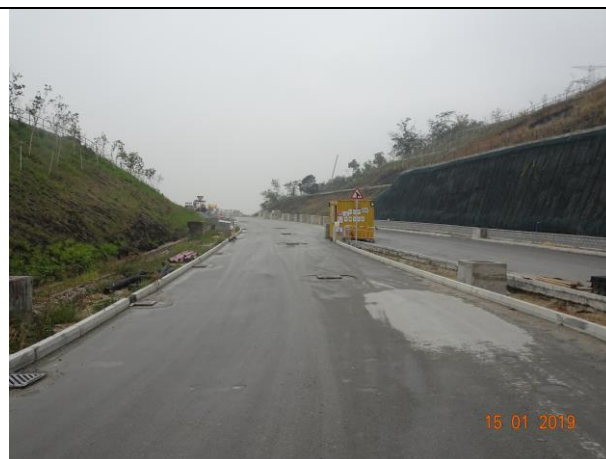
Photo 8 Water spraying was observed at site haul road during the joint site inspection on 15 January 2019.
