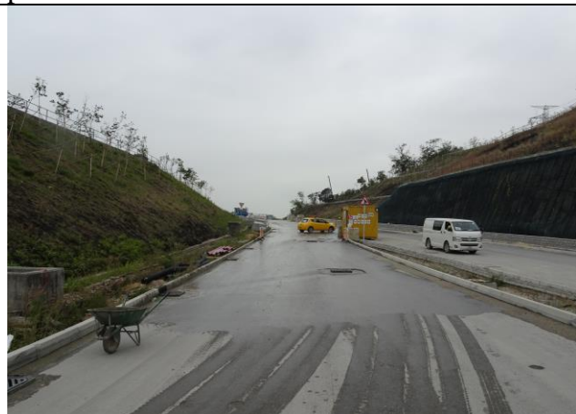
Photo 9 Water spraying was observed at site haul road during the joint site inspection on 8 January 2019.
