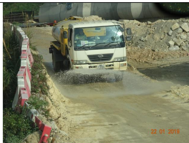
Photo 8 Water spraying was observed at site haul road during the joint site inspection on 22 January 2019.
