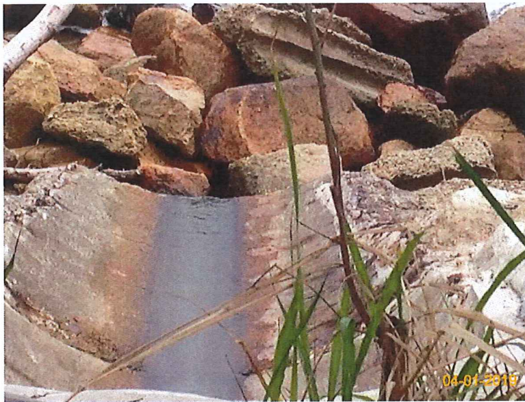
Item 7. Ensure no run-off into water body.(Outfall 1)
