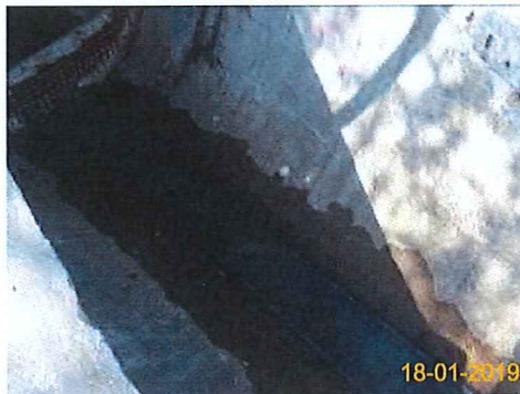
Item 7. Ensure no run-off into water body.(Outfall 1)
