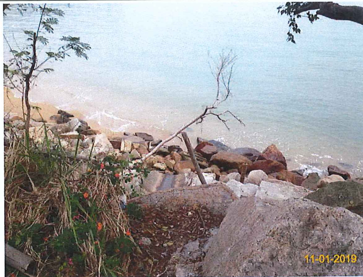
Item 7. Ensure no run-off into water body.(Outfall 1)
