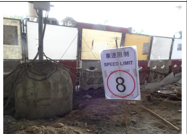
Photo 6 All vehicles using the haul road had enhanced to control the speed below 8km/hr to reduce dust emission.
