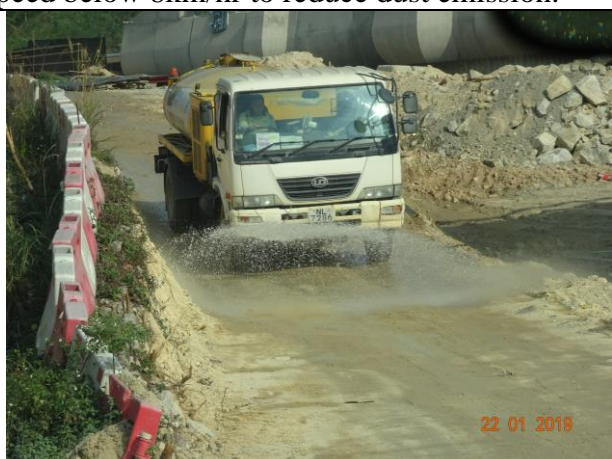
Photo 9 Water spraying was observed at site haul road during the joint site inspection on 22 January 2019.
