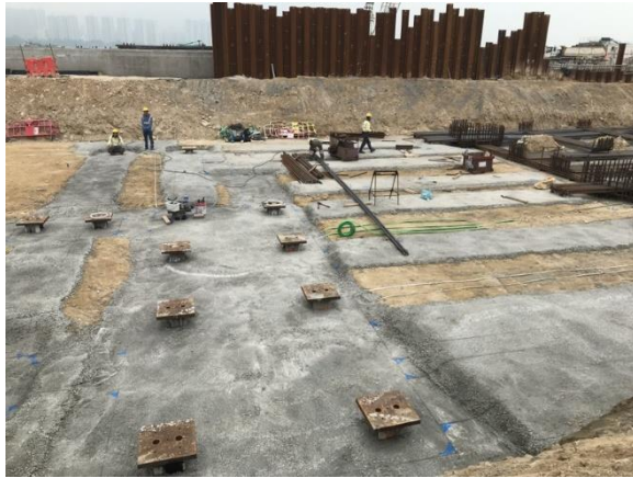
Photo 1 - Rebar fixing conducted at works area of Administration Building and Maintenance Depot
