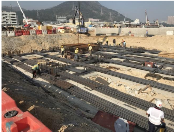
Photo 1 - Rebar fixing conducted at works area of Administration Building and Maintenance Depot
