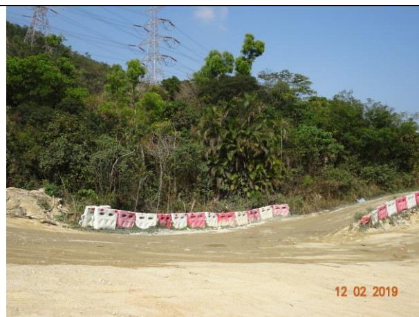
Photo 8 Water spraying was observed at site haul road during the joint site inspection on 12 February 2019.
