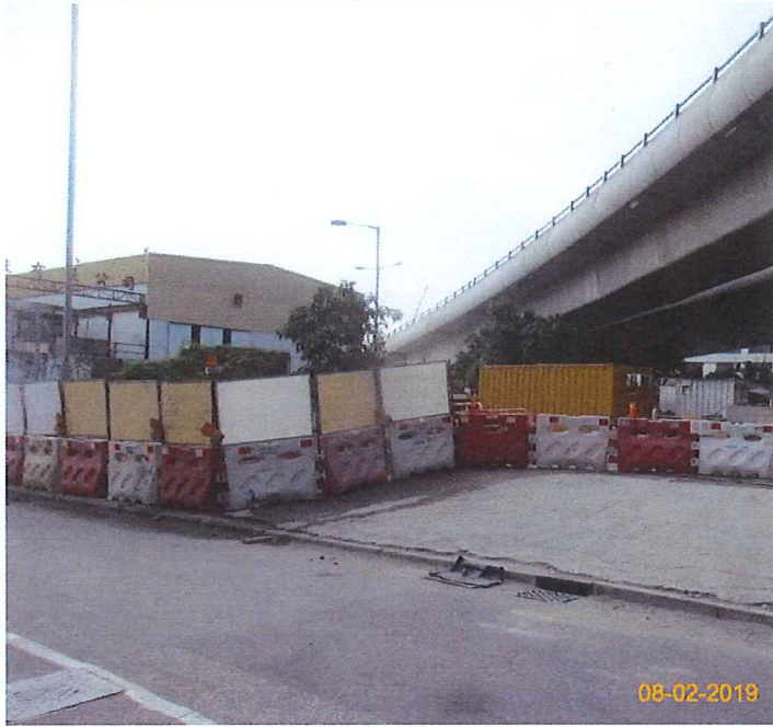
Item 5. Hoarding with panel around works area & Item 6. Temporary traffic management lighting.
