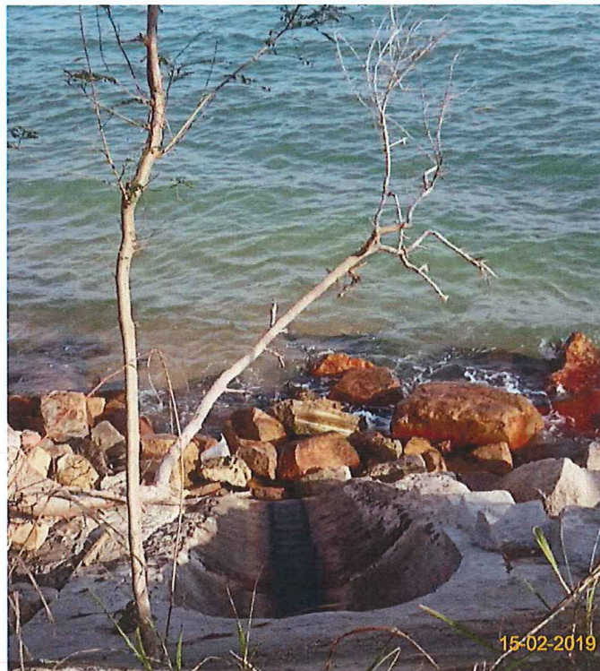
Item 7. Ensure no run-off into water body.(Outfall 1)
