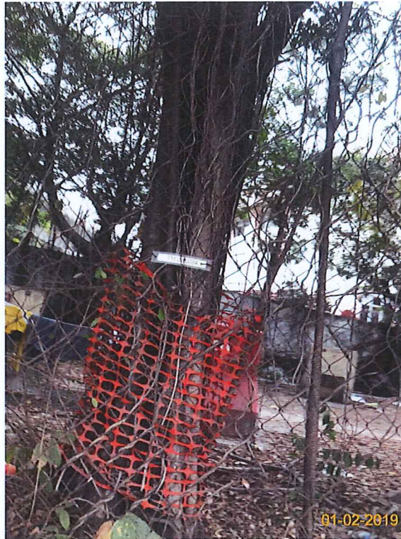
Item 1. Existing trees on boundary of the Project Area should be protected carefully during construction.
