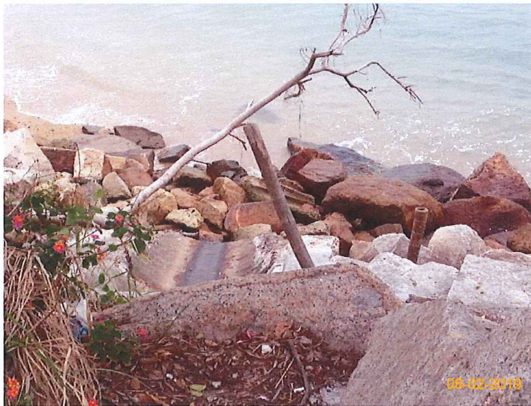
Item 7. Ensure no run-off into water body.(Outfall 1)
