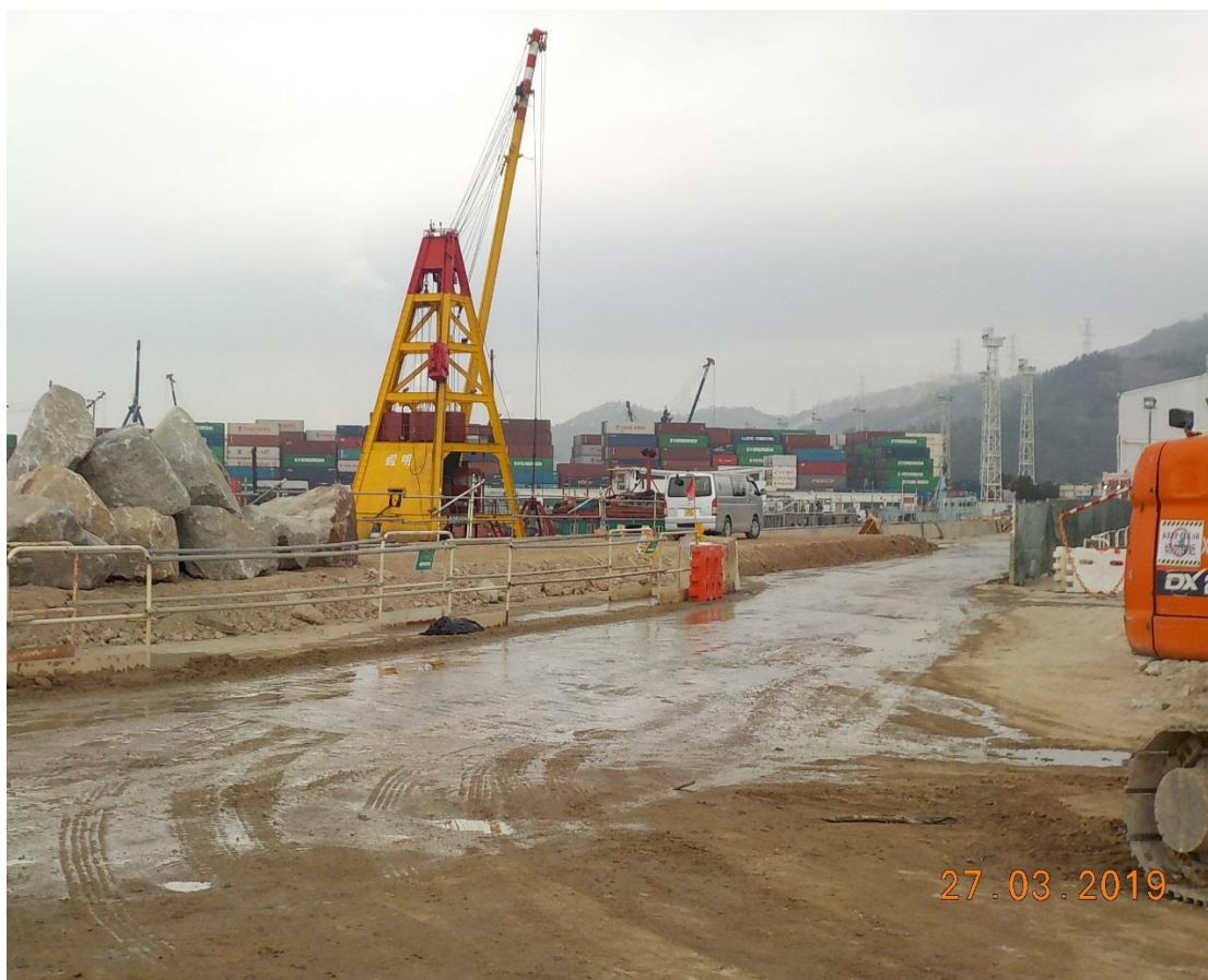
Water spraying was applied at the main haul road to prevent dust. (Works Area Portion N-A)
