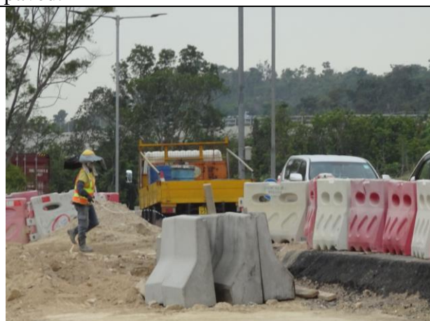
Photo 10 Water spraying was observed at works area during the joint site inspection on 4 April 2019.
