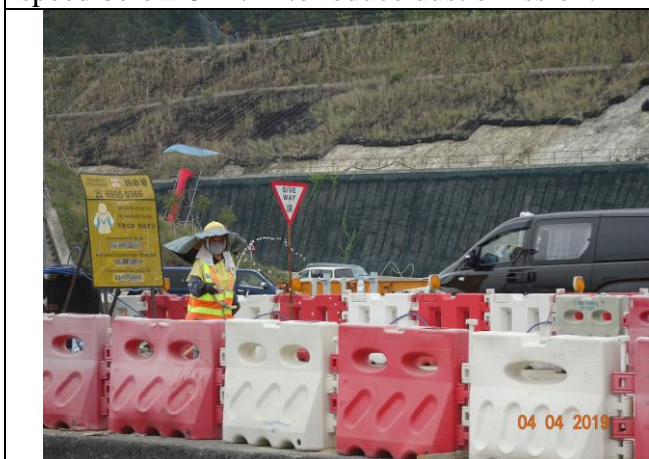
Photo 9 Water spraying was observed at works area during the joint site inspection on 4 April 2019.
