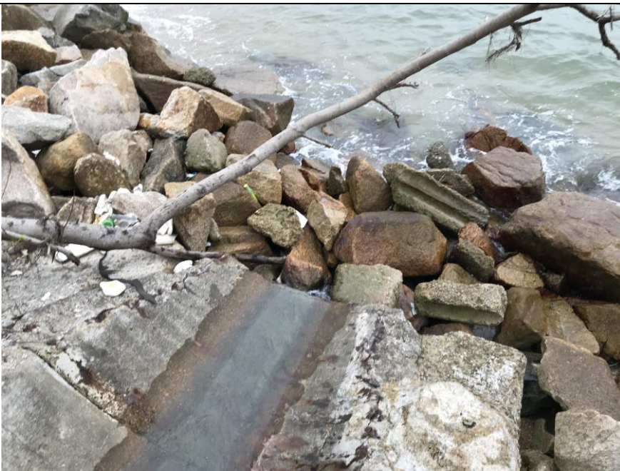
Outfall 1: Clean water is discharging.
