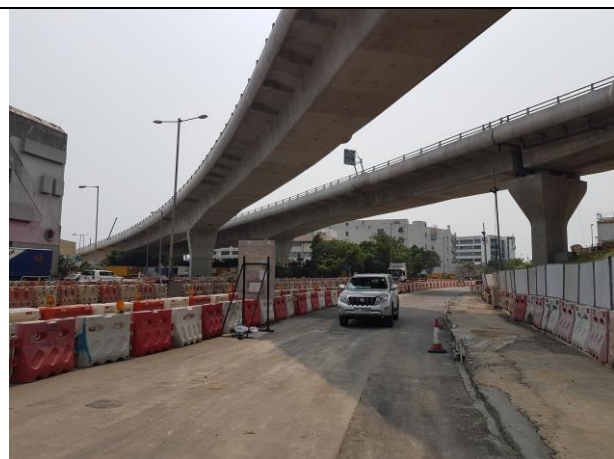
Photo 8 During the joint site inspection on 26 March 2019 most of the site area was hard paved.
