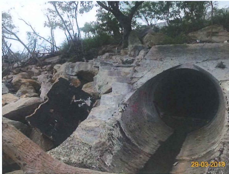
Item 7. Ensure no run-off into water body.(Outfall 1)
