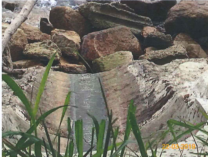
Item 7. Ensure no run-off into water body.(Outfall 1)
