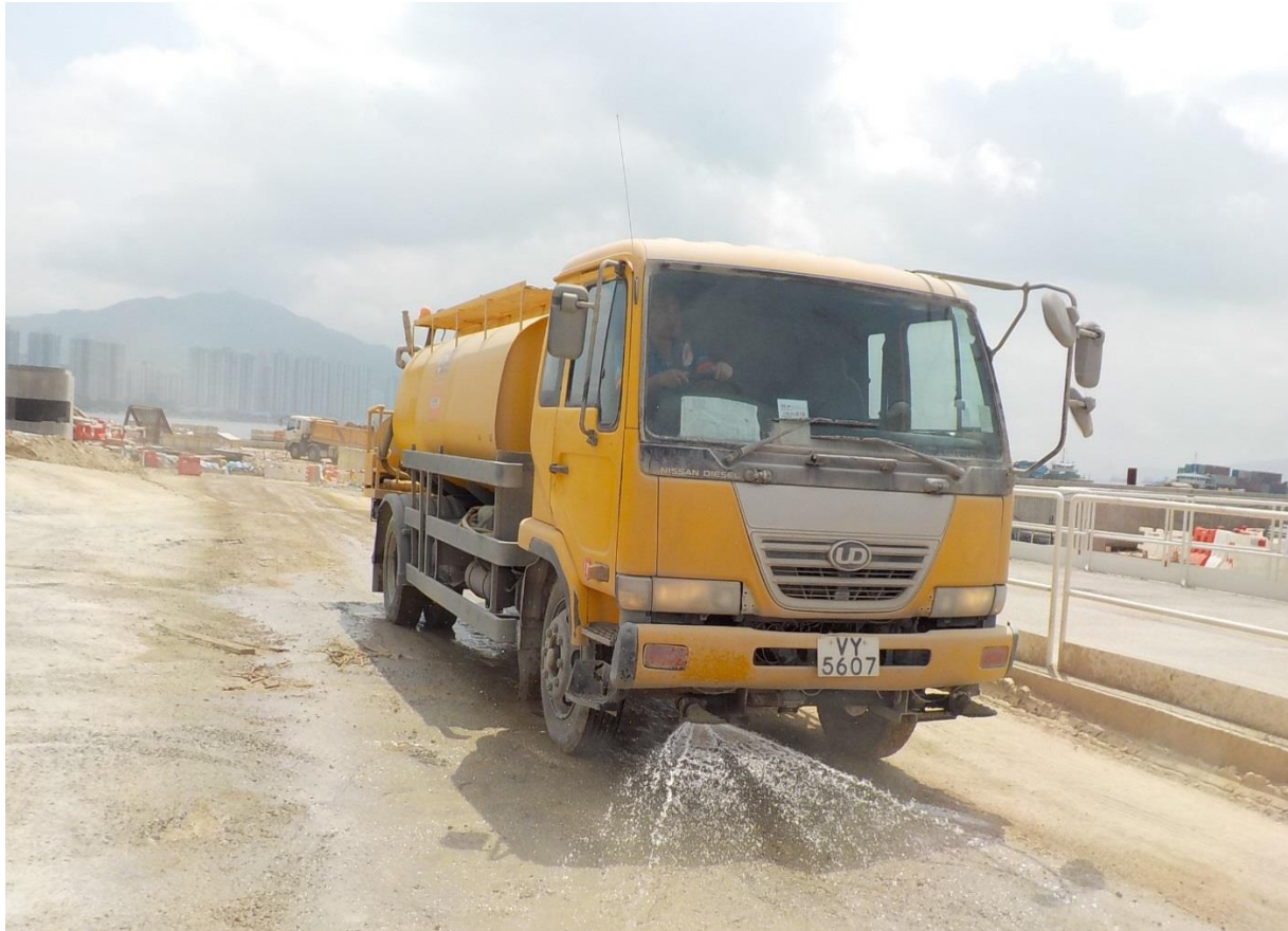
Water spraying was applied at the main haul road to prevent dust. (Works Area Portion N-C)
