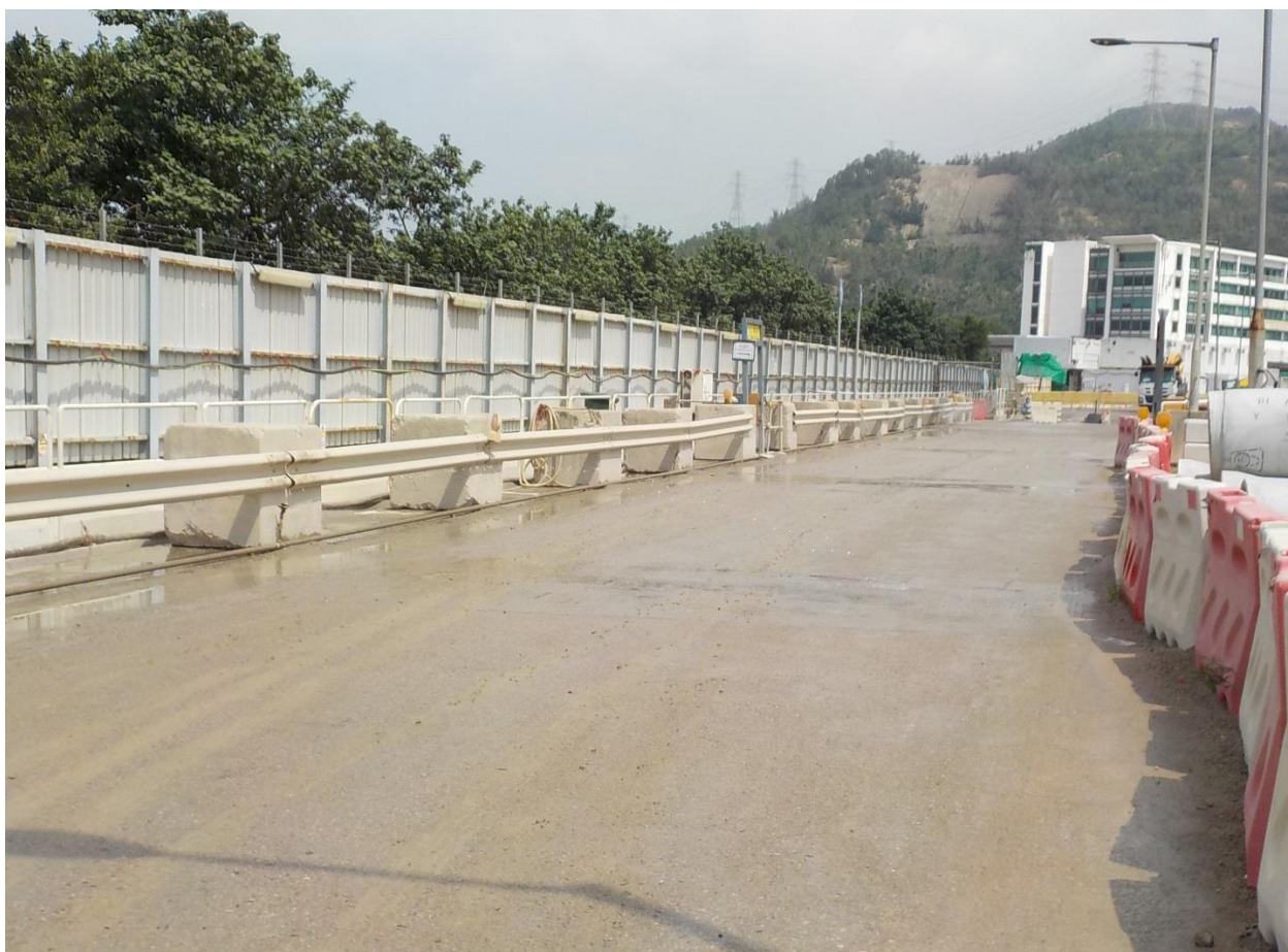
Water spraying was applied at the main haul road to prevent dust. (Works Area Portion N-A)
