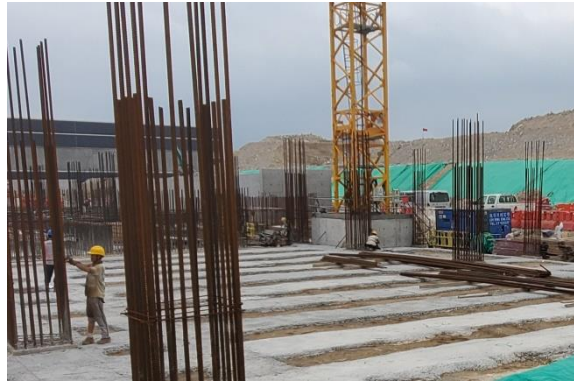
Photo 2- Building structure was conducted at works area of Customs and Excise Building (24 May 2019)
