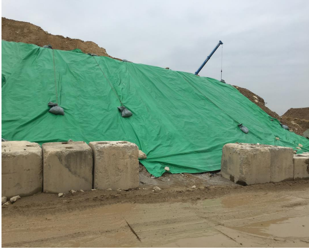
Exposed soil was covered by tarpaulin sheet to prevent dust. (Works Area Portion N-C)
