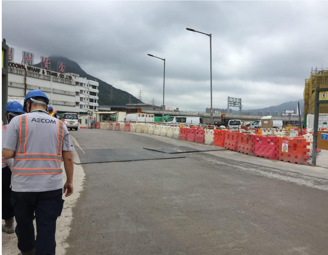
Water spraying was applied on main haul road near Chu Kong Warehouse.
