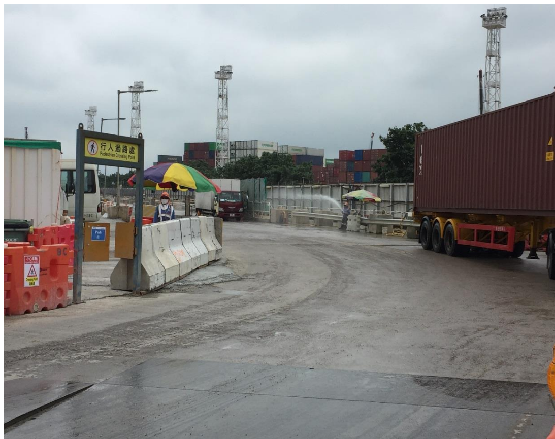
Water spraying was applied on main haul road near Chu Kong Warehouse.
