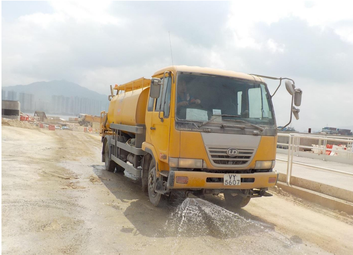
Water spraying was applied at the main haul road to prevent dust. (Works Area Portion N-C)
