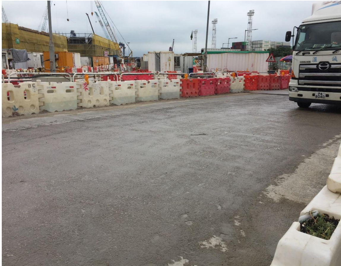
Water spraying was applied on main haul road near Chu Kong Warehouse.
