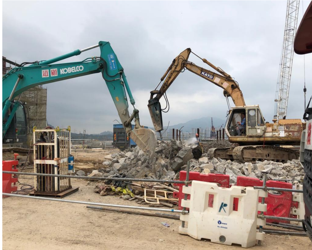
Water spraying was applied during rock breaking to prevent dust. (Works Area Portion N-A)
