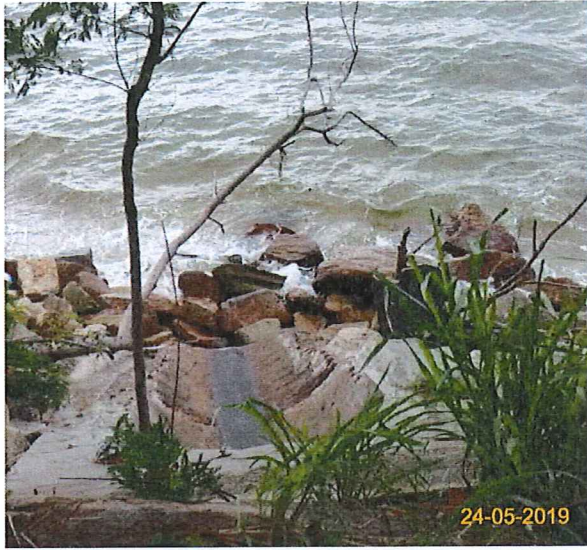
Item 7. Ensure no run-off into water body.(Outfall 1)
