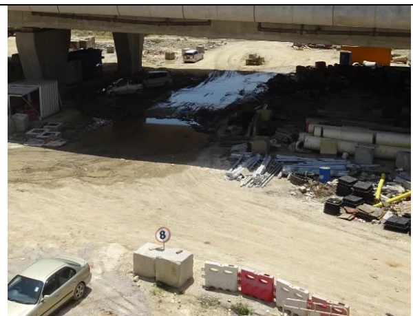
Photo 6 All vehicles using the haul road had enhanced to control the speed below 8km/hr to reduce dust emission.
