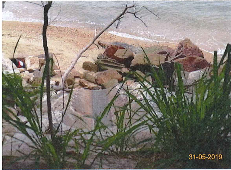
Item 7. Ensure no run-off into water body.(Outfall 1)
