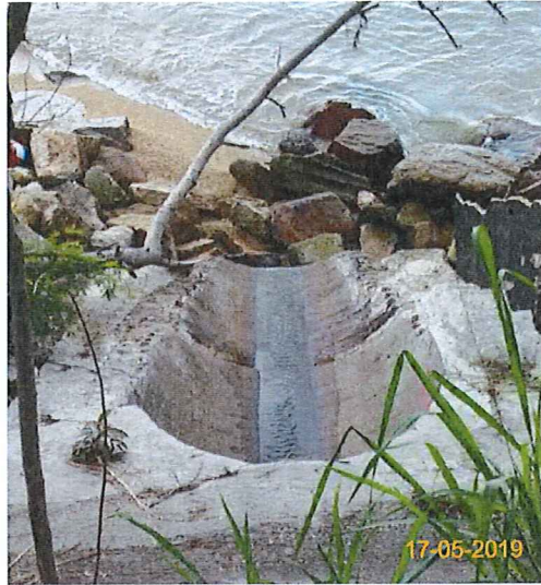
Item 7. Ensure no run-off into water body.(Outfall 1)
