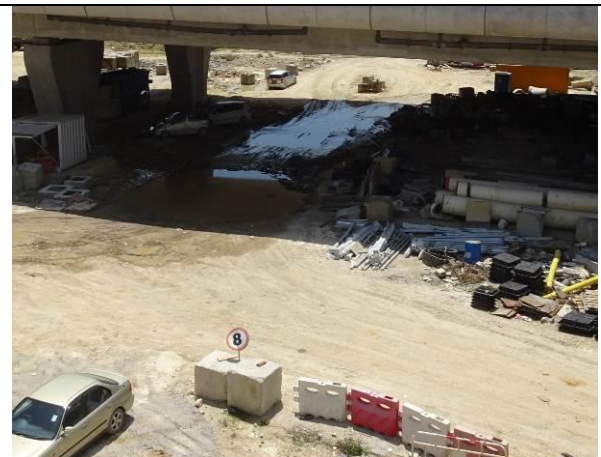
Photo 6 All vehicles using the haul road had enhanced to control the speed below 8km/hr to reduce dust emission.
