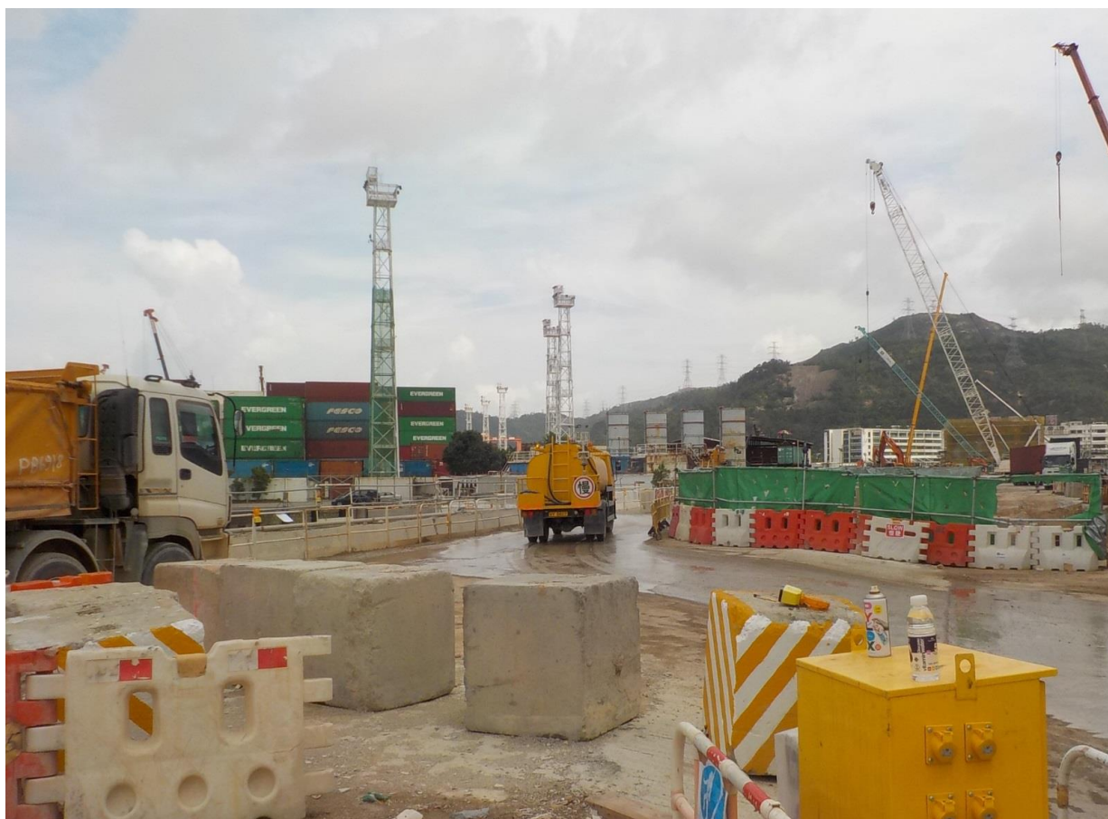
Water truck was used for water spraying to prevent dust. (Works Area Portion N-A)
