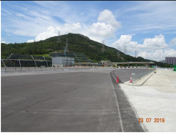
Photo 7 During the joint site inspection on 23 July 2019 most of the site area was hard paved.
