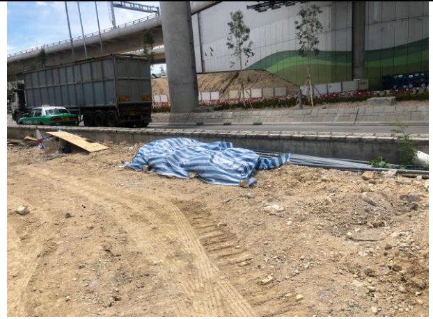
Photo 8 During the joint site inspection on 30 July 2019 stockpile storage on site was covered with tarpaulin.
