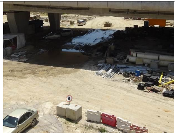
Photo 4 All vehicles using the haul road had enhanced to control the speed below 8km/hr to reduce dust emission.
