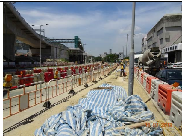
Photo 10 During the joint site inspection on 16 July 2019 stockpile storage on site was covered with tarpaulin.
