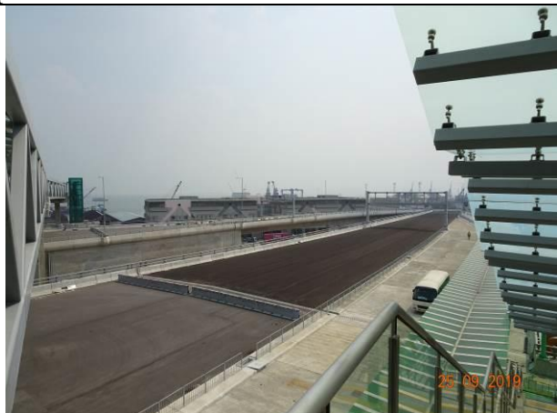
Photo 9 During the joint site inspection on 25 September 2019 most of the site area was hard paved.
