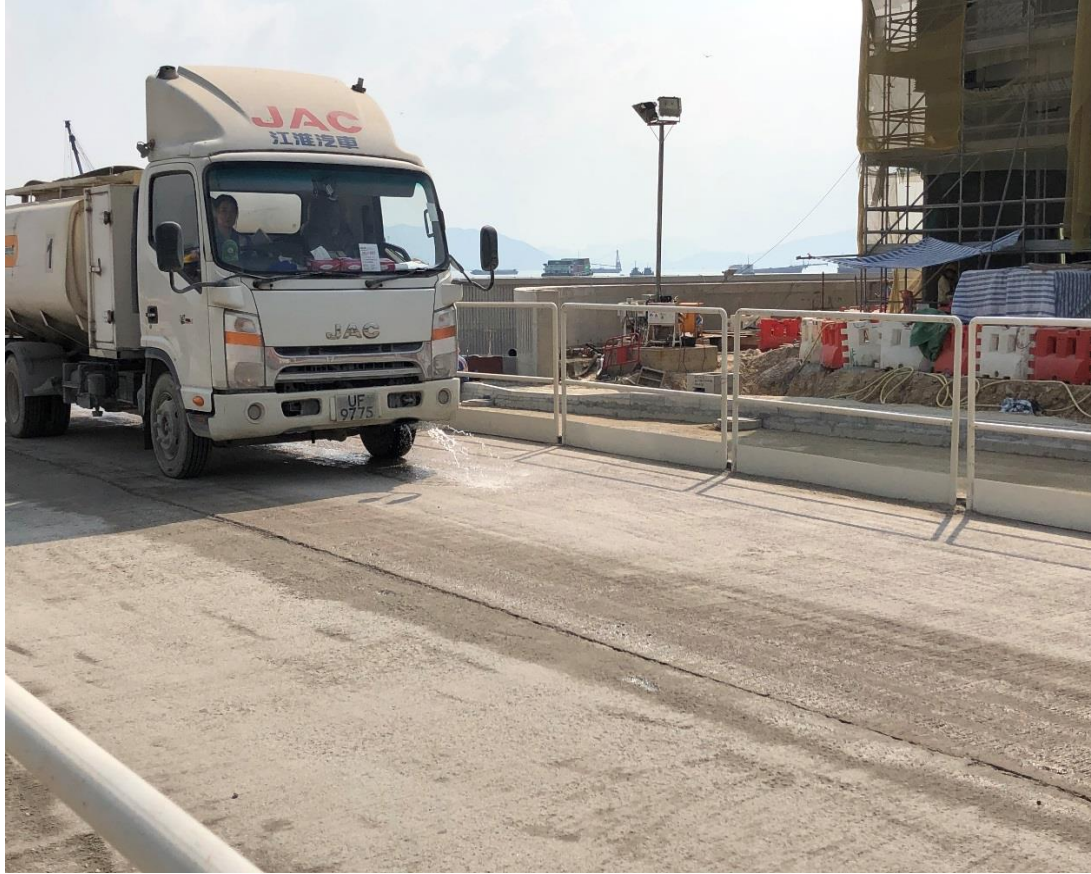
Water truck was used for water spraying to prevent dust. (Works Area Portion N-C)
