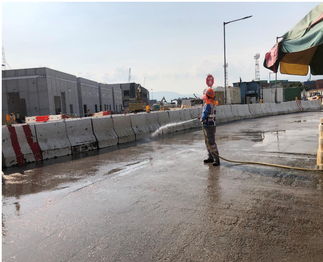
Water spraying was applied on main haul road to prevent dust. (Works Area Portion N-A)
