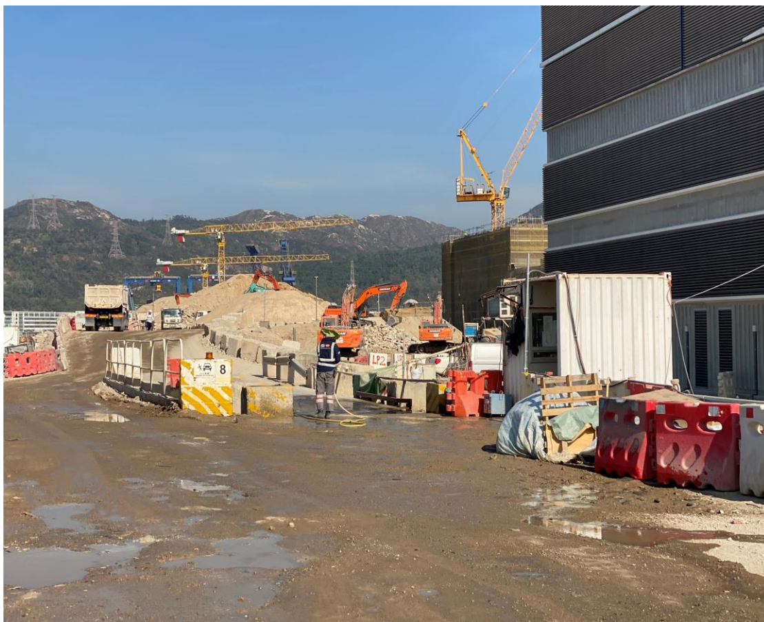
Water spraying was applied on main haul road to prevent dust. (Works Area Portion N-C)
