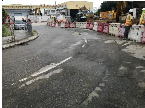
Photo 10 During the joint site inspection on 15 October 2019 water spraying was provided for the exposed surface to reduce dust impact.
