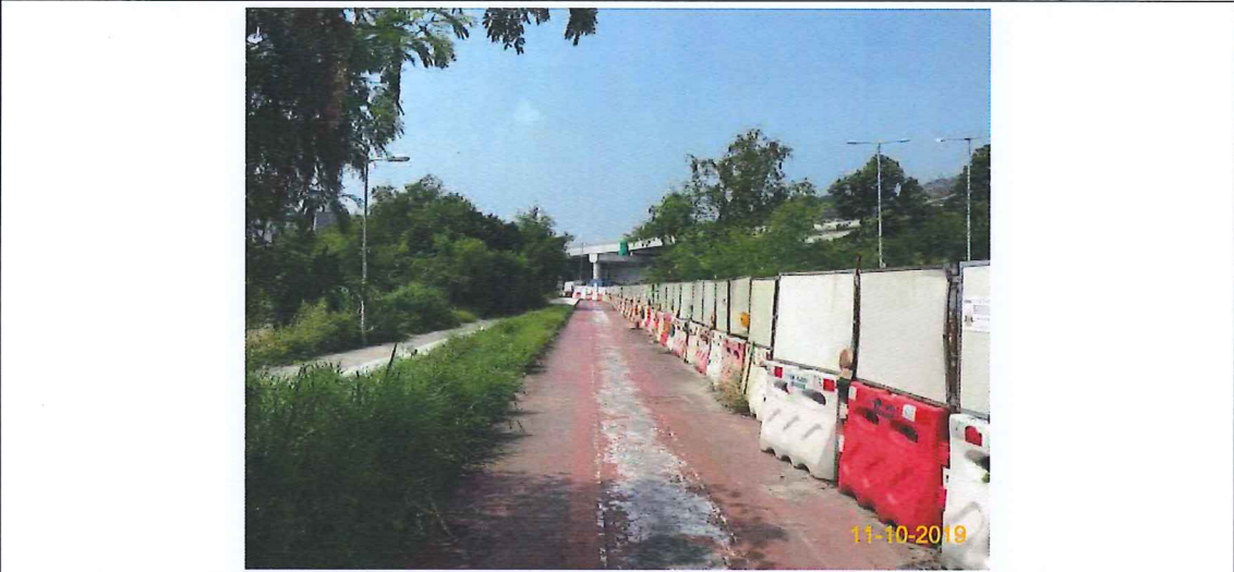
Item 5. Hoarding with panel around works area & Item 6. Temporary traffic management lighting.
