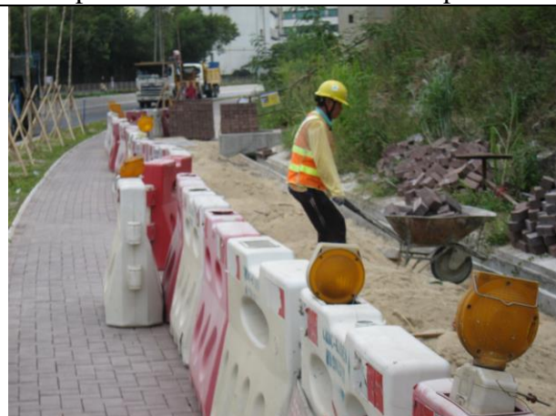
Photo 12 Paving block in pedestrian road at Lung Mun Road
