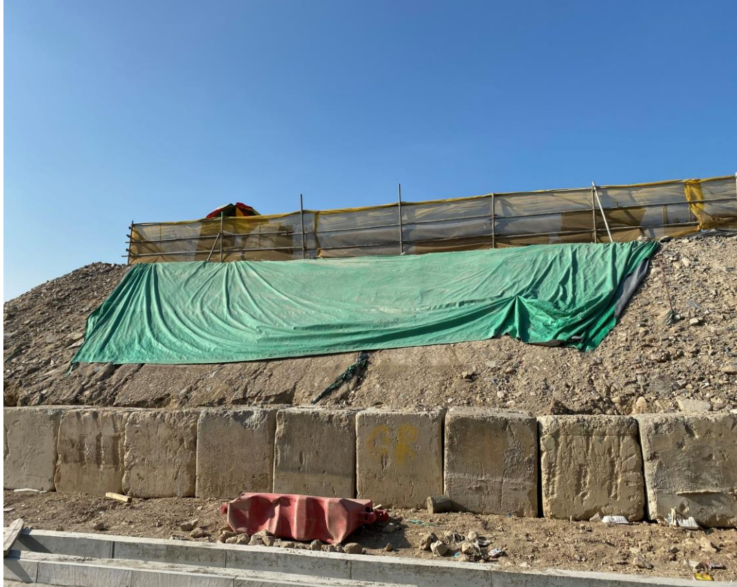
Exposed soil is covered by tarpaulin sheet to prevent dust. (Works Area Portion N-C)
