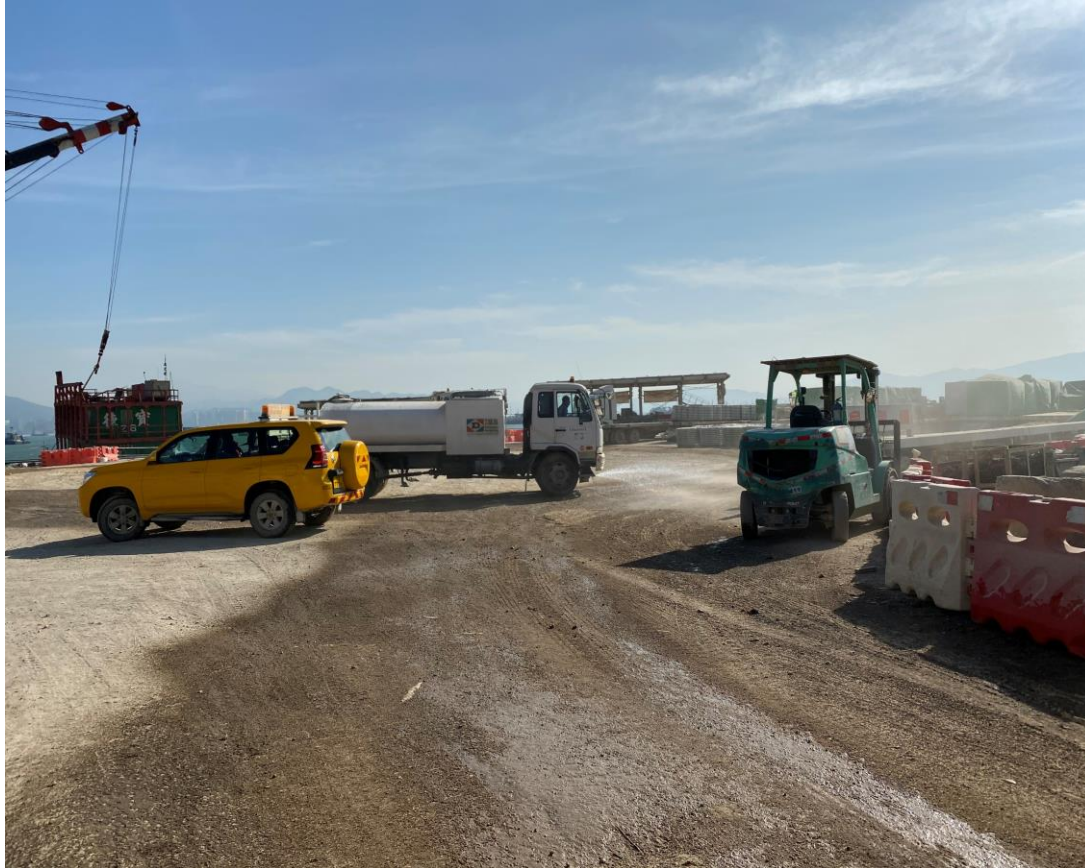
Water truck was used for water spraying to prevent dust. (Works Area Portion N-A)
