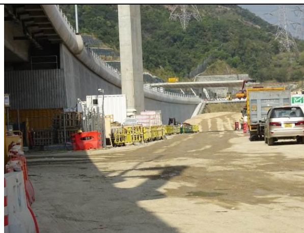
Photo 8 During the joint site inspection on 5 November 2019 water spraying had been provided for the haul road to reduce dust impact.
