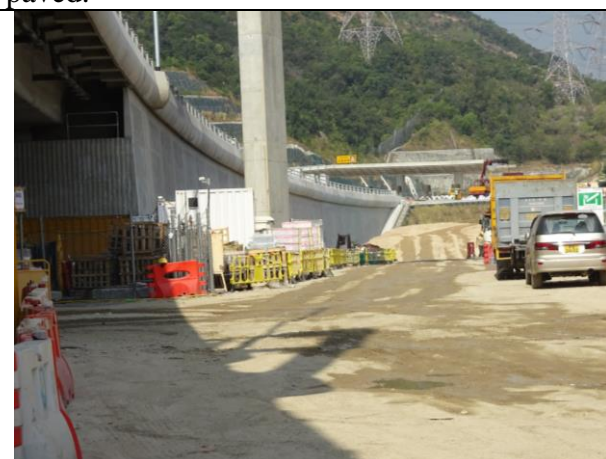
Photo 10 During the joint site inspection on 5 November 2019 water spraying had been provided for the haul road to reduce dust impact.
