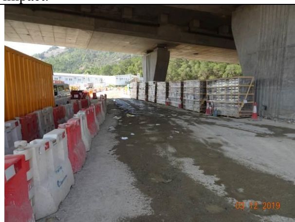
Photo 10 During the joint site inspection on 3 December 2019 water spraying had been provided for the haul road to reduce dust impact.
