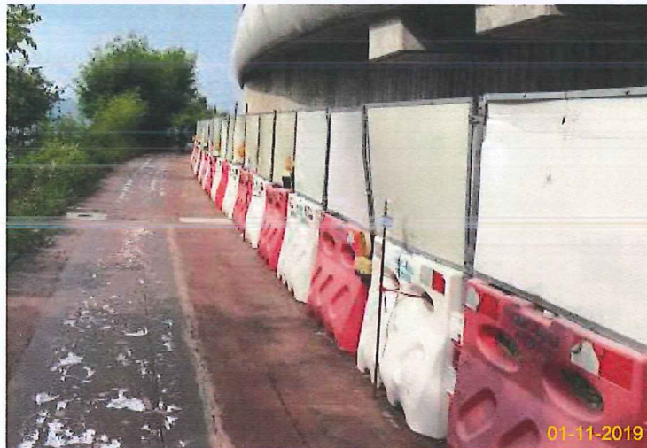
Item 5. Hoarding with panel around works area & Item 6. Temporary traffic management lighting.
