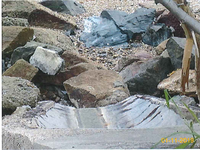
Item 7. Ensure no run-off into water body.(Outfall 1)
