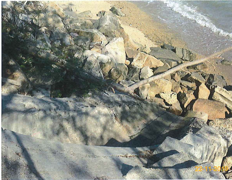
Item 7. Ensure no run-off into water body.(Outfall 1)
