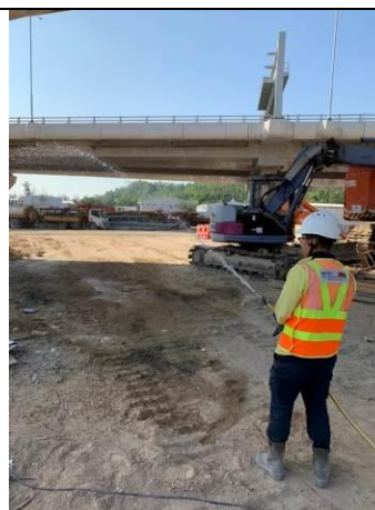
Photo 8 During the joint site inspection on 26 November 2019 water spraying had been provided for the exposed area to reduce dust impact.
