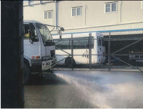
Photo 1 Watering of haul road by water truck to keep road surface wet
