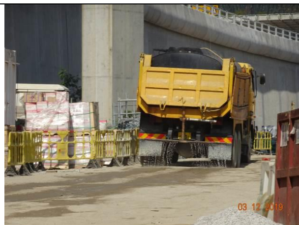
Photo 8 During the joint site inspection on 3 December 2019 water spraying had been provided for the haul road to reduce dust impact.
