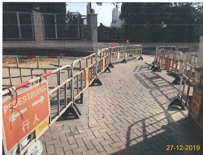
Item 6. Temporary traffic management lighting.
