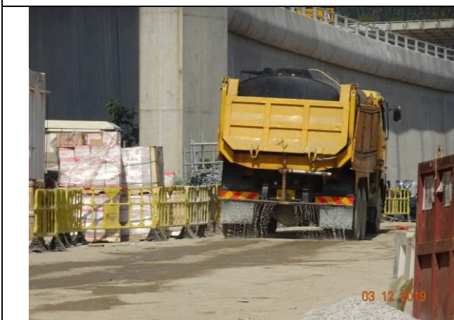
Photo 9 During the joint site inspection on 3 December 2019 water spraying had been provided for the haul road to reduce dust impact.
