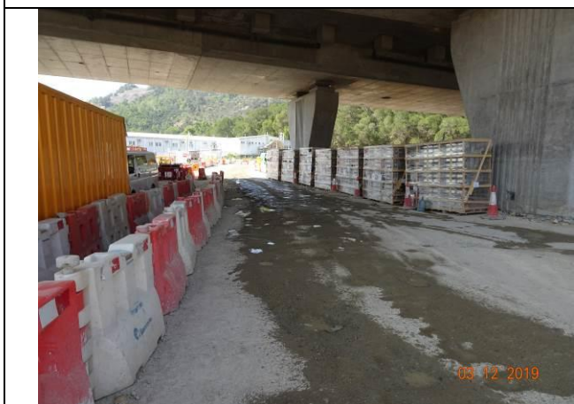
Photo 9 During the joint site inspection on 3 December 2019 water spraying had been provided for the haul road to reduce dust impact.
