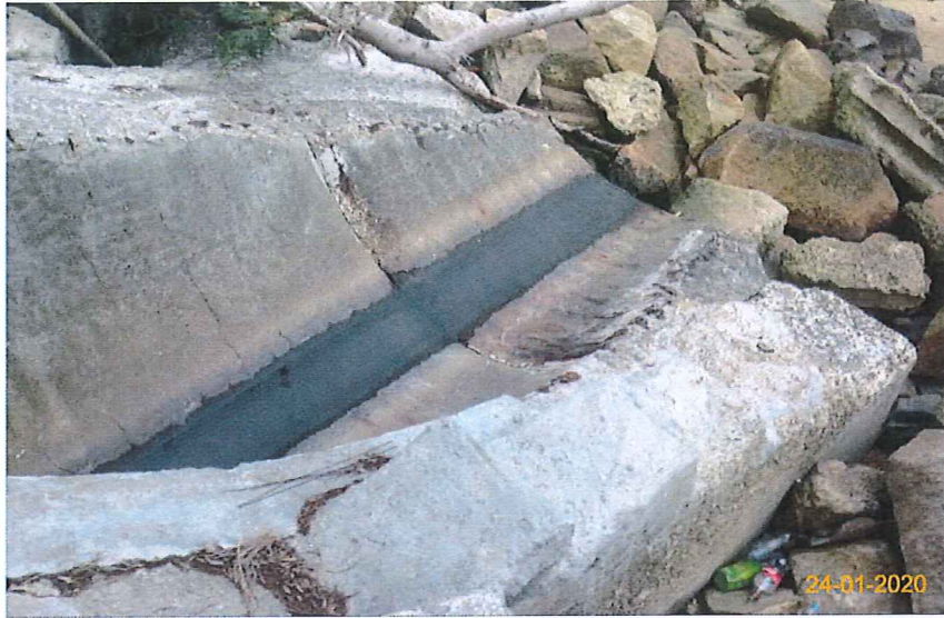
Item 7. Ensure no run-off into water body.(Outfall 1)
