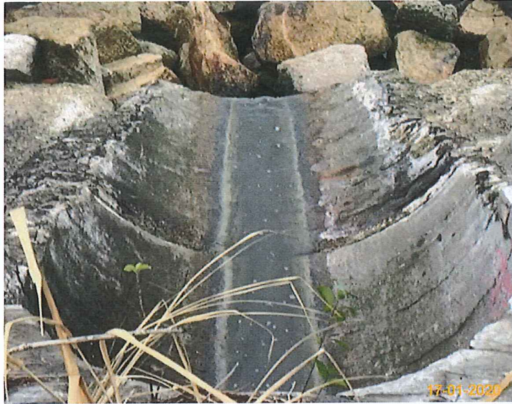
Item 7. Ensure no run-off into water body.(Outfall 1)
