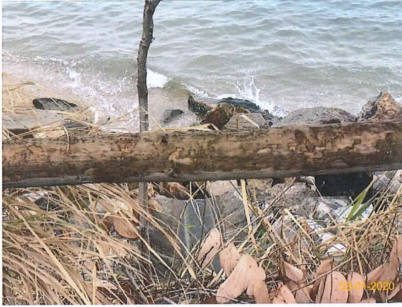
Item 7. Ensure no run-off into water body.(Outfall 1)
