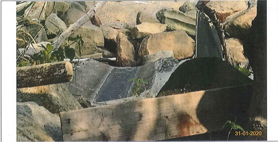
Item 7. Ensure no run-off into water body.(Outfall 1)
