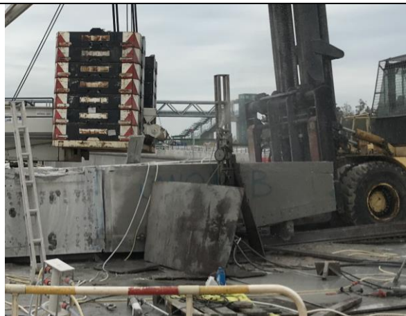
Photo 9 During the joint site inspection on 14 April 2020 water spraying had been provided for the toll booth modification works to reduce dust impact.
