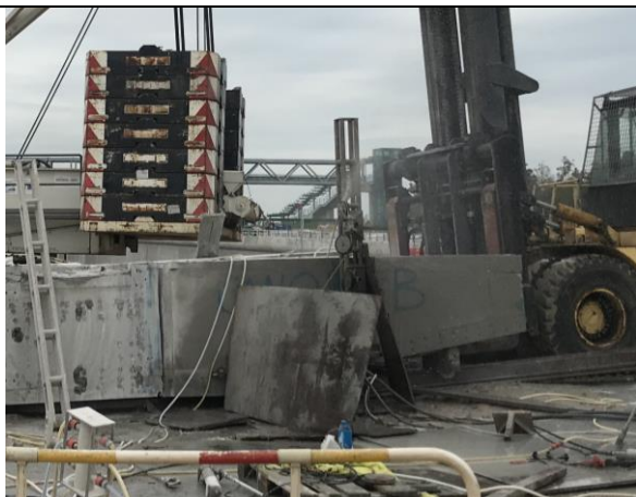
Photo 9 During the joint site inspection on 14 April 2020 water spraying had been provided for the toll booth modification works to reduce dust impact.
